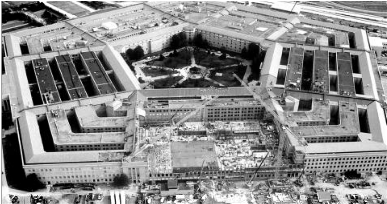
PENTAGON RENOVATION PROGRAM: Around-the-clock efforts by thousands of workers have put the reconstruction of the 60-year-old Pentagon ahead of schedule, and more than 2,000 employees have already returned to their desks in the damaged section. The completed structure will be dedicated on September 11, 2002.
