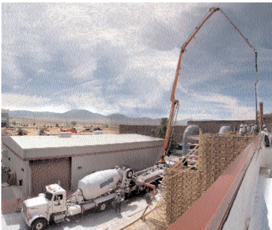
MESA TAKES SHAPE — A construction crew manages an 80-yard concrete pour for a Specialty Gas Room at the east end of the Microelectronics Development Laboratory. The vitally important MESA project has met several milestones over the past year.
