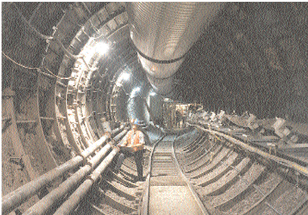
GETTING THE DRIFT — An engineer at the Yucca Mountain project in Nevada checks out a tunnel at the proposed nuclear waste repository. Sandia researchers are helping understand the mechanics of rock structure in new areas of the project.
