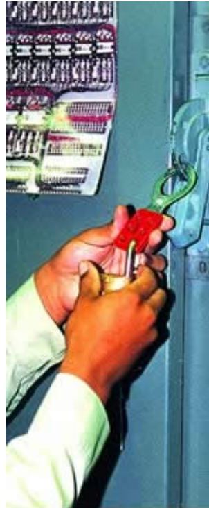
This worker is applying a group lock-out device. The equipment cannot be re-started until all workers remove their locks.
