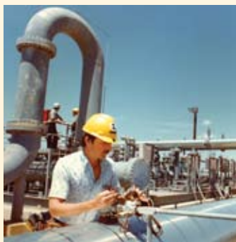
SPR worker checks pumps.
