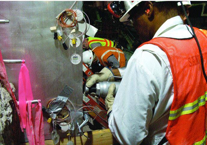
Sandia workers install a flat-jack into a slot in the Yucca Mountain rock. Experimenters studied the effects of expanding pressure on the volcanic tuff of the mountain.
