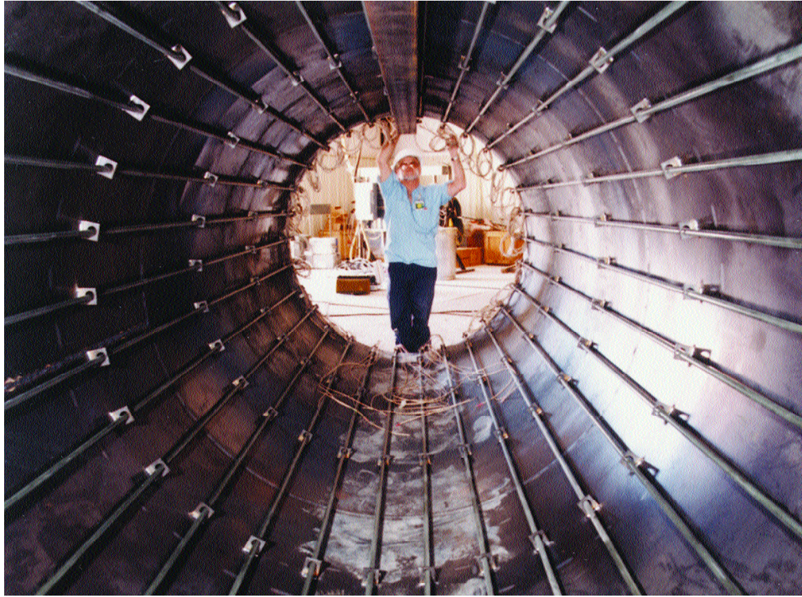
Yucca Mountain worker adjusts heater assembly during construction for the drift scale test. Heater simulated spent fuel rods.
