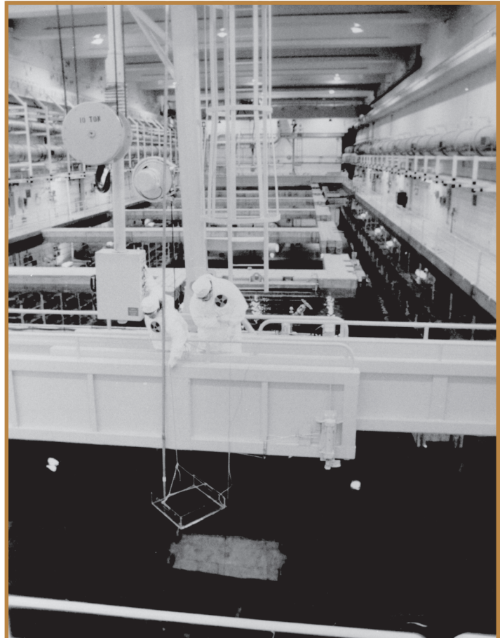
Shown is a view of workers inside the Idaho Chemical Processing Plant.
