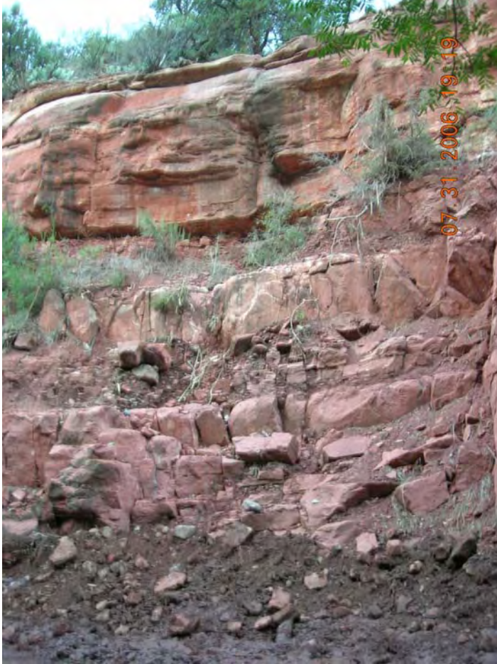
DSCN 1584: Rock slide and sediment debris, location ~ M.P. 77.8, just north of Trout Farm about 300 feet. Didn't hike above the sandstone ledge but the immediate area above the rock outcrop was unburned and out of the fire perimeter. There is a concavity in the outcrop where much of the rock failed. The probable cause of the rock fall was concentration of water running over the top of the ledge loosening up the rock and soil along preexisting fractures. The lower part of the outcrop area is highly fractured. Need to recon the slopes above the ledge to see if channels were formed where the water concentrated up slope and if the burned area above was a factor. The upper part of the rock outcrop shows a water mark staining where water has flown before. The rock and mud piled up over the guard railing and flowed over into Oak Creek – see picture below.
