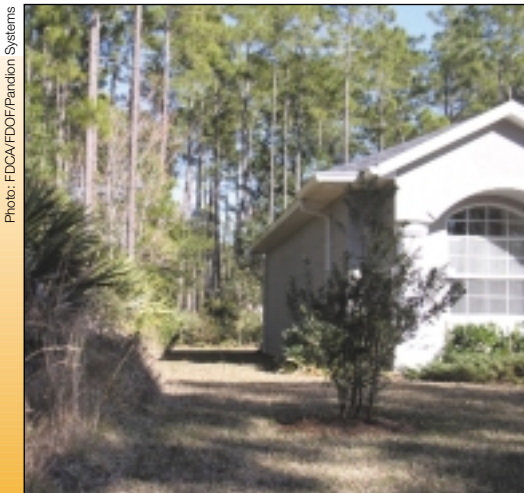
This wildland-urban interface home has a heavy fuel load near the side yard.
