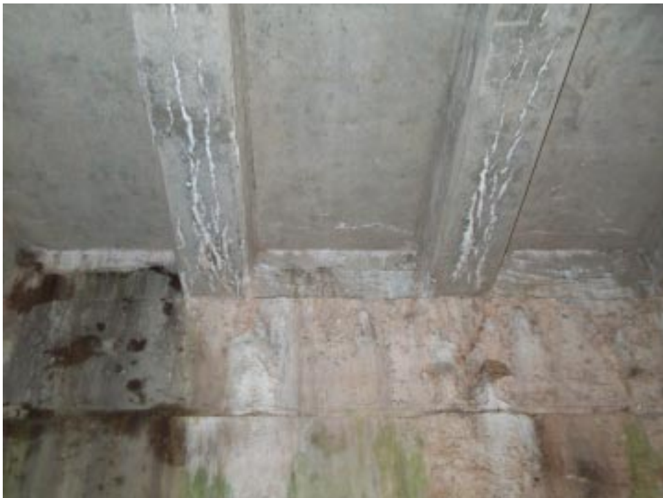
Figure 112. Deterioration described by Note B3 – T-beam deterioration.
