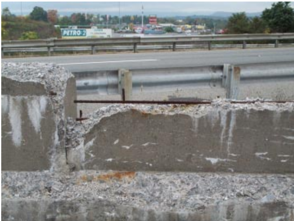
Figure 118. Deterioration described by Note D2 – Severe parapet deterioration.
