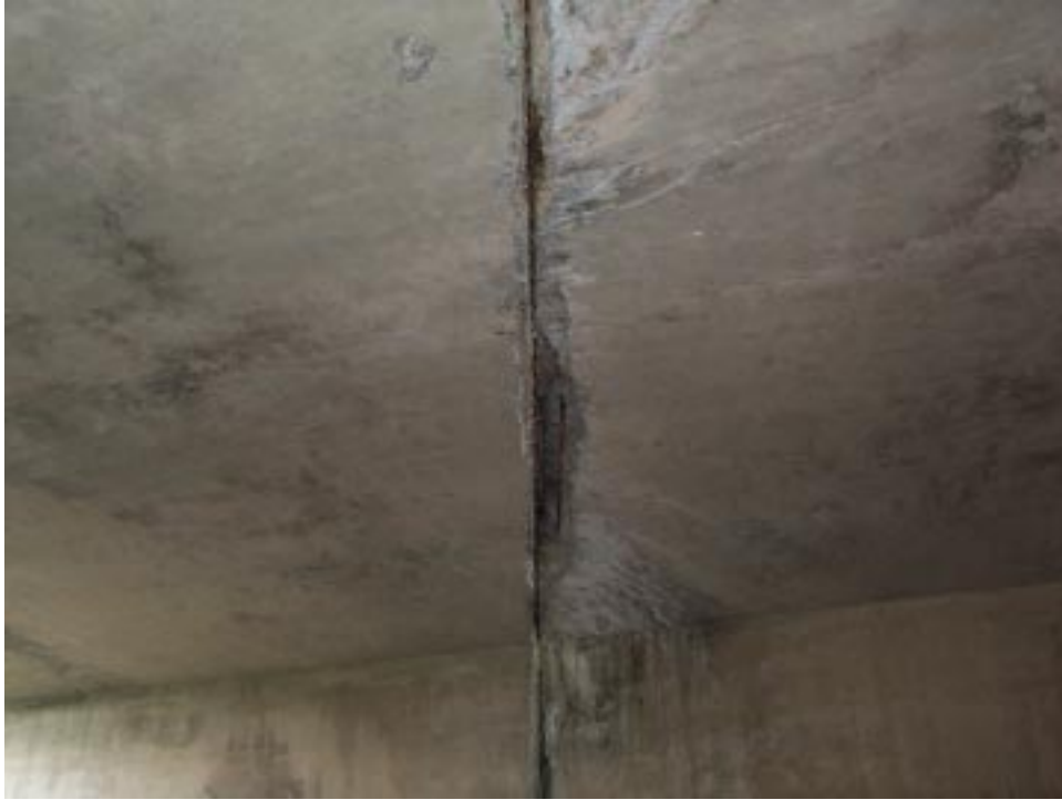
Figure 119. Deterioration described by Note D3 – Longitudinal joint deterioration.
