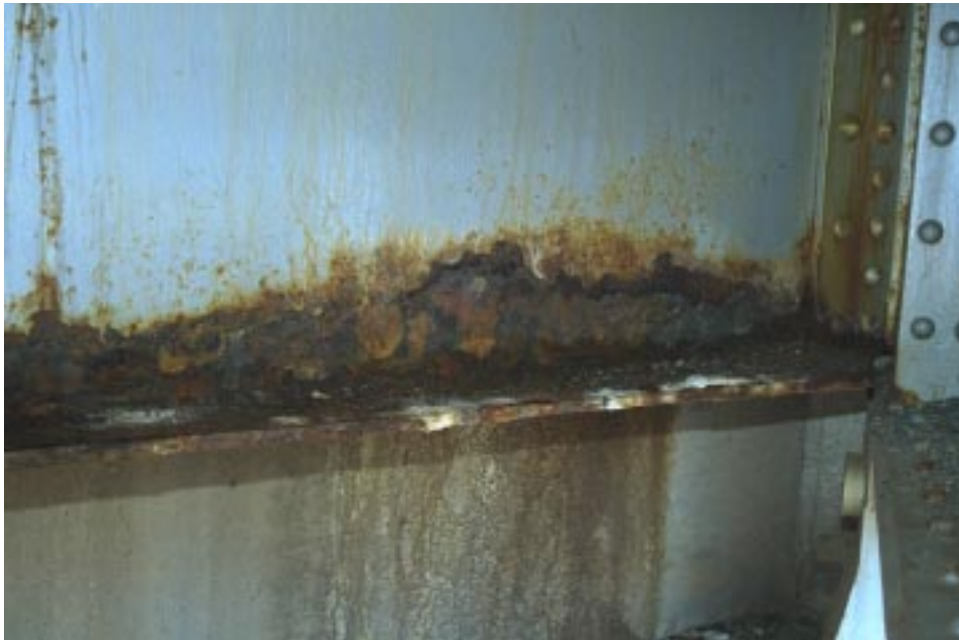
Figure 106. Deterioration described by Note A2 – Heavy corrosion of end floor beam.
