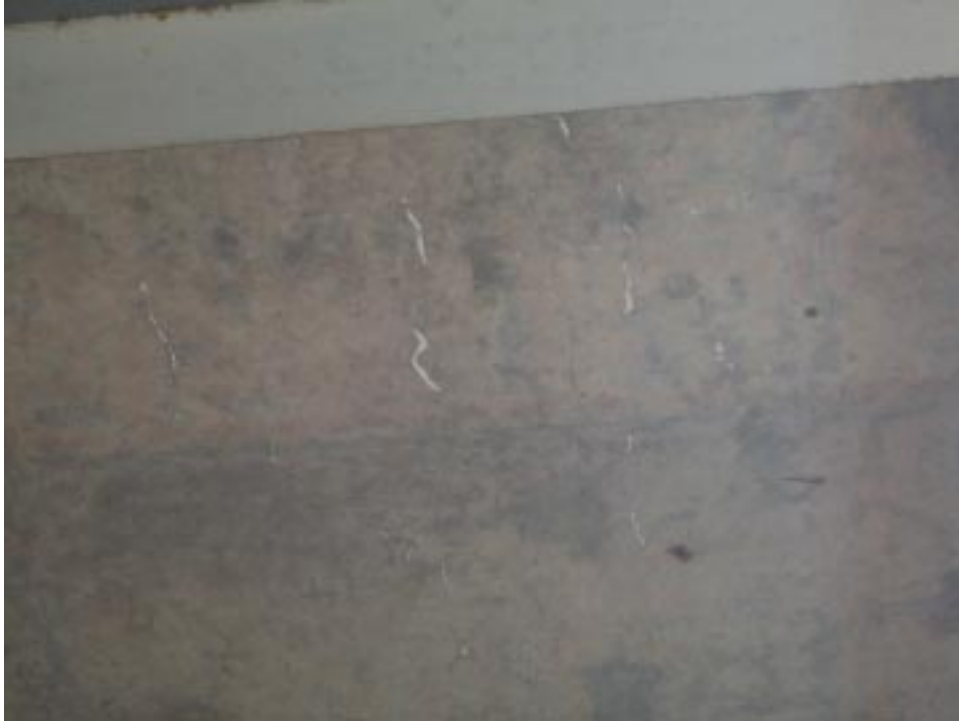
Figure 105. Deterioration described by Note A1 – Underside deck cracking and/or efflorescence.
