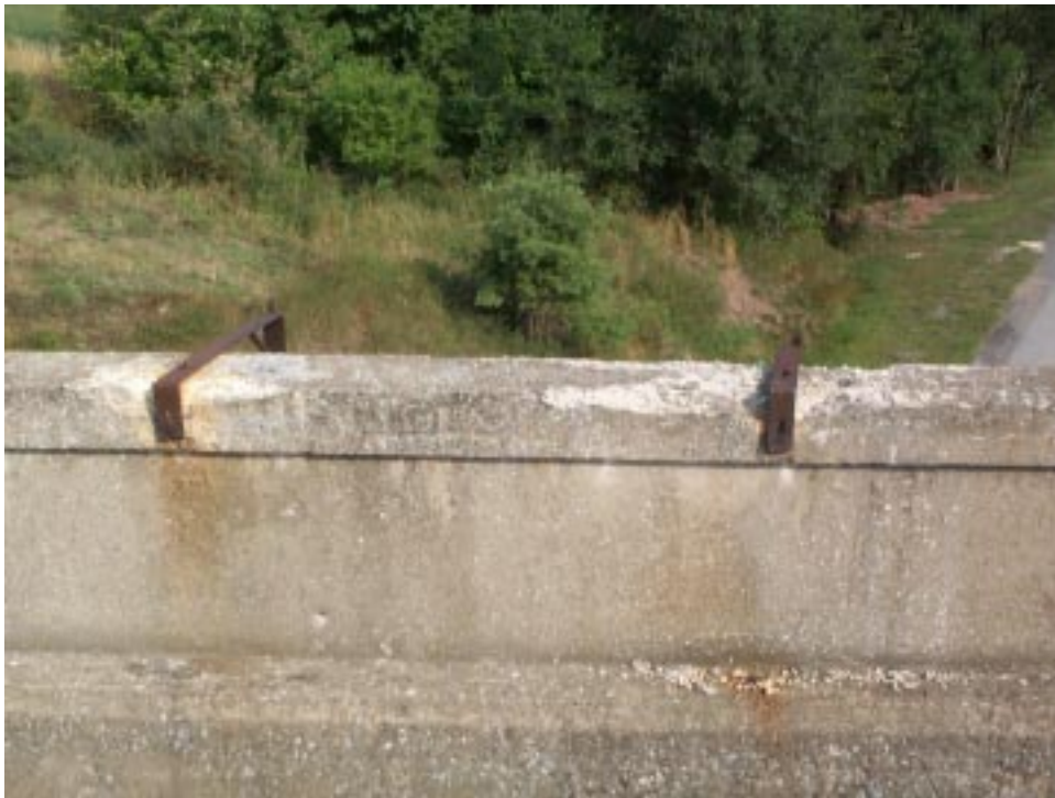
Figure 92. Inspector Photograph 6 – Failed overhead sign connection.
