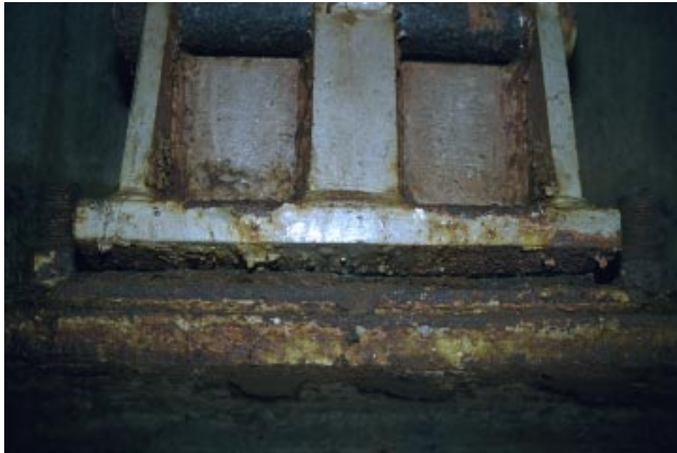
Figure 124. Deterioration described by Note G1 – Moderate to severe corrosion of abutment bearings.
