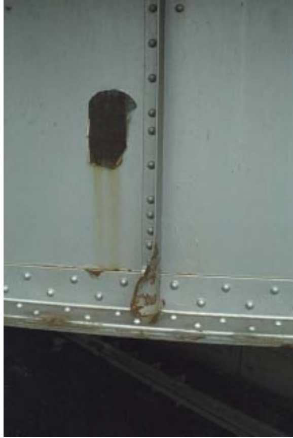
Figure 123. Deterioration described by Note E4 – Impact damage to south fascia girder.
