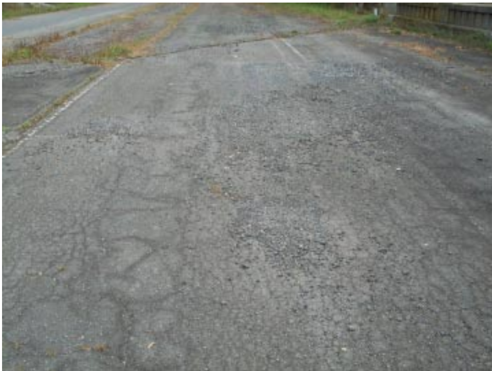
Figure 120. Deterioration described by Note E1 – Severe deterioration of wearing surface.
