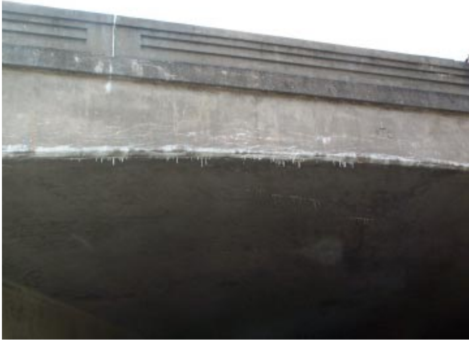
Figure 87. Inspector Photograph 1 – Longitudinal cracking in southern face of superstructure.
