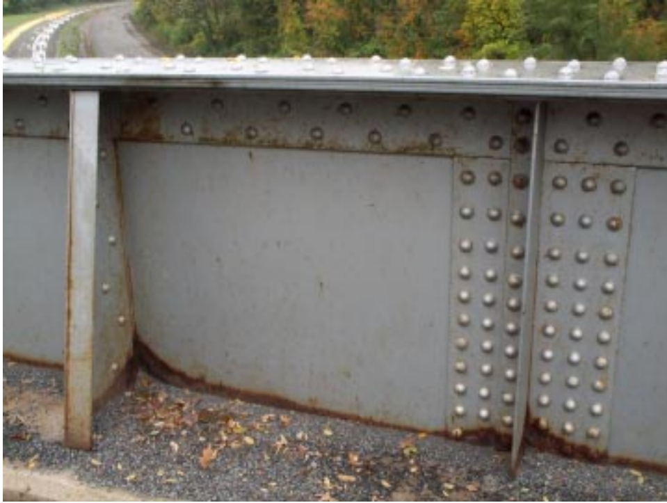
Figure 107. Deterioration described by Note A3 – Minor to moderate corrosion of stringer web at deck interface.
