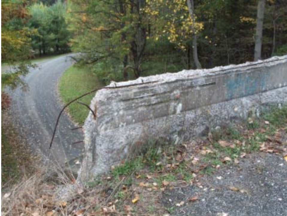
Figure 111. Deterioration described by Note B2 – Severe parapet deterioration.
