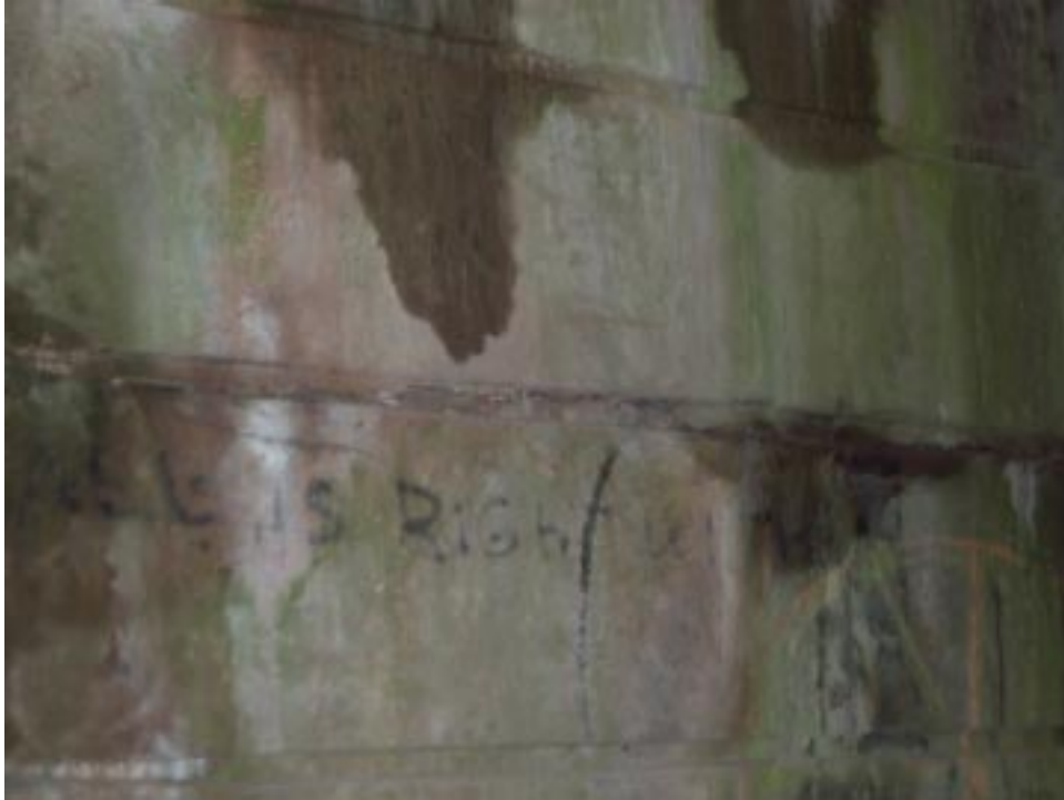
Figure 113. Deterioration described by Note B4 – Full-length horizontal crack.
