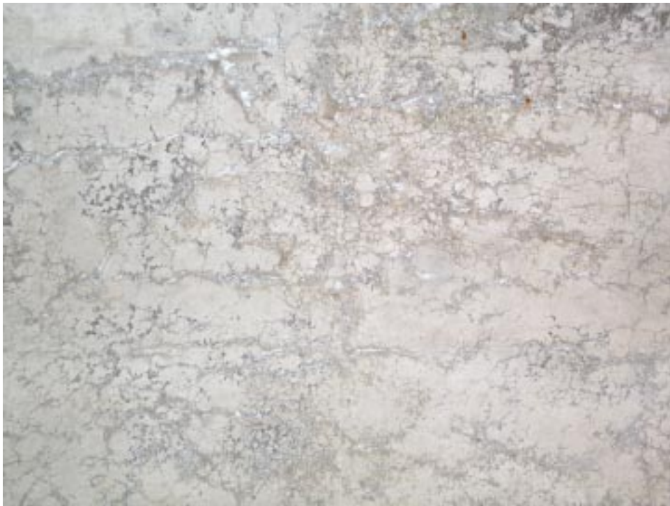
Figure 88. Inspector Photograph 2 – Typical underside deck cracking.
