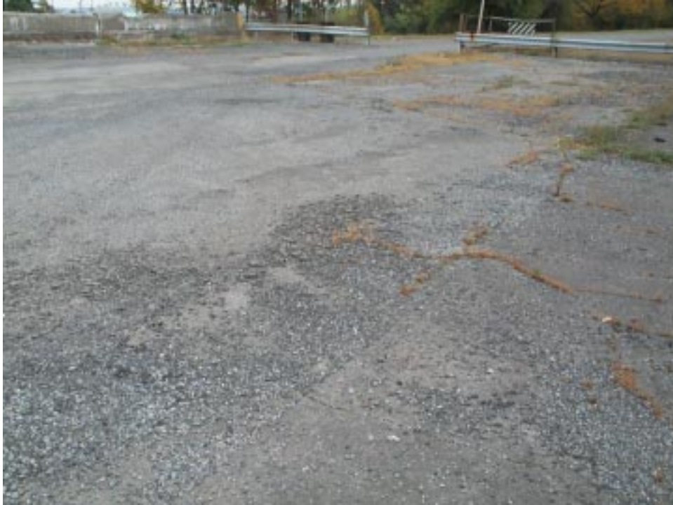
Figure 117. Deterioration described by Note D1 – Severe deterioration of wearing surface.
