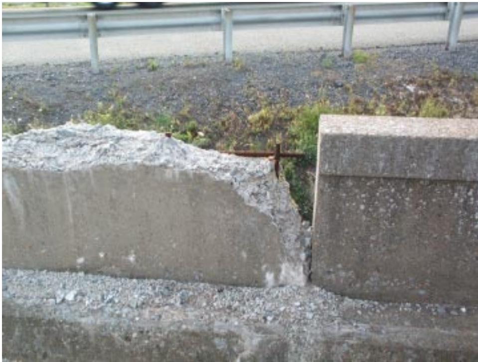
Figure 94. Inspector Photograph 8 – Typical parapet concrete deterioration and exposed reinforcement.
