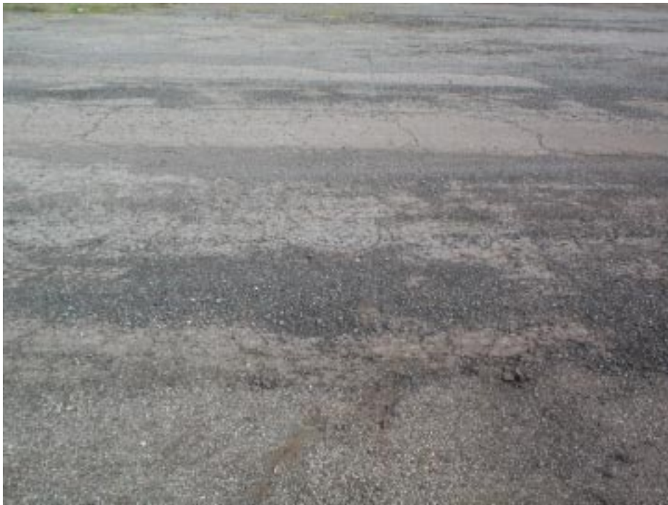
Figure 96. Inspector Photograph 10 – Typical wearing surface deterioration.
