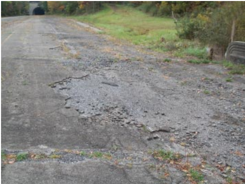
Figure 114. Deterioration described by Note C1 – Severe deterioration of wearing surface.
