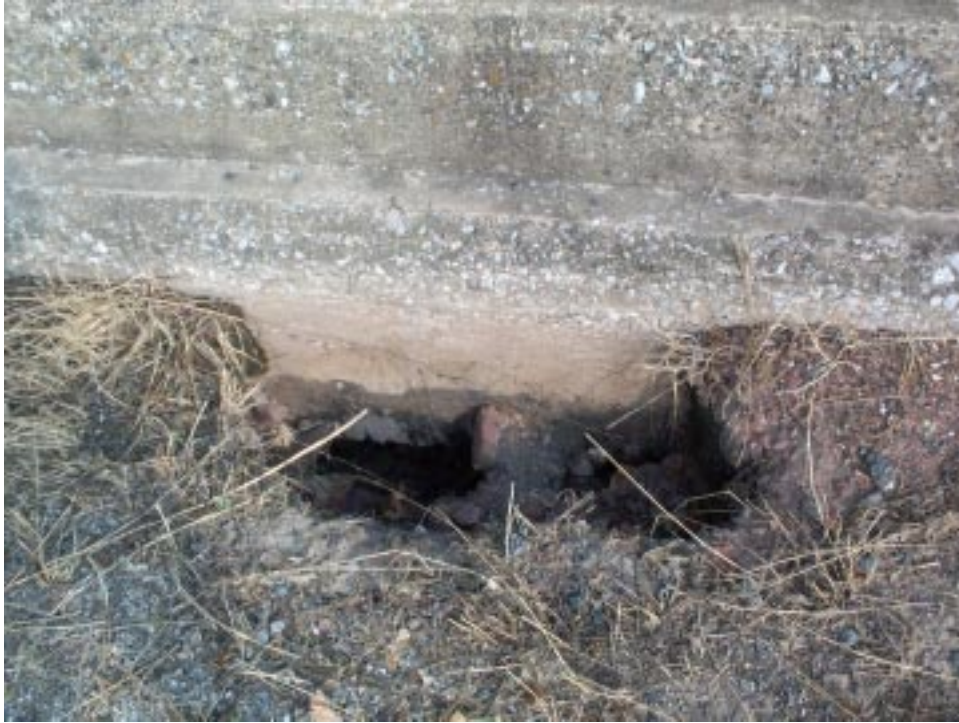
Figure 93. Inspector Photograph 7 – Hole in east approach.
