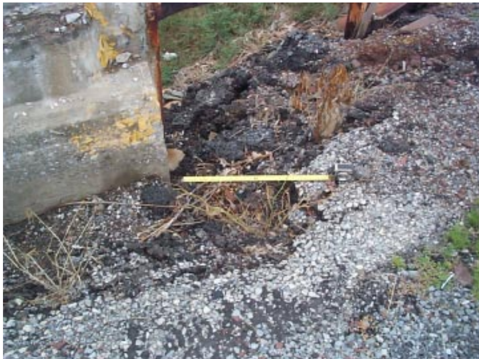
Figure 104. Inspector Photograph 18 – Localized soil erosion.
