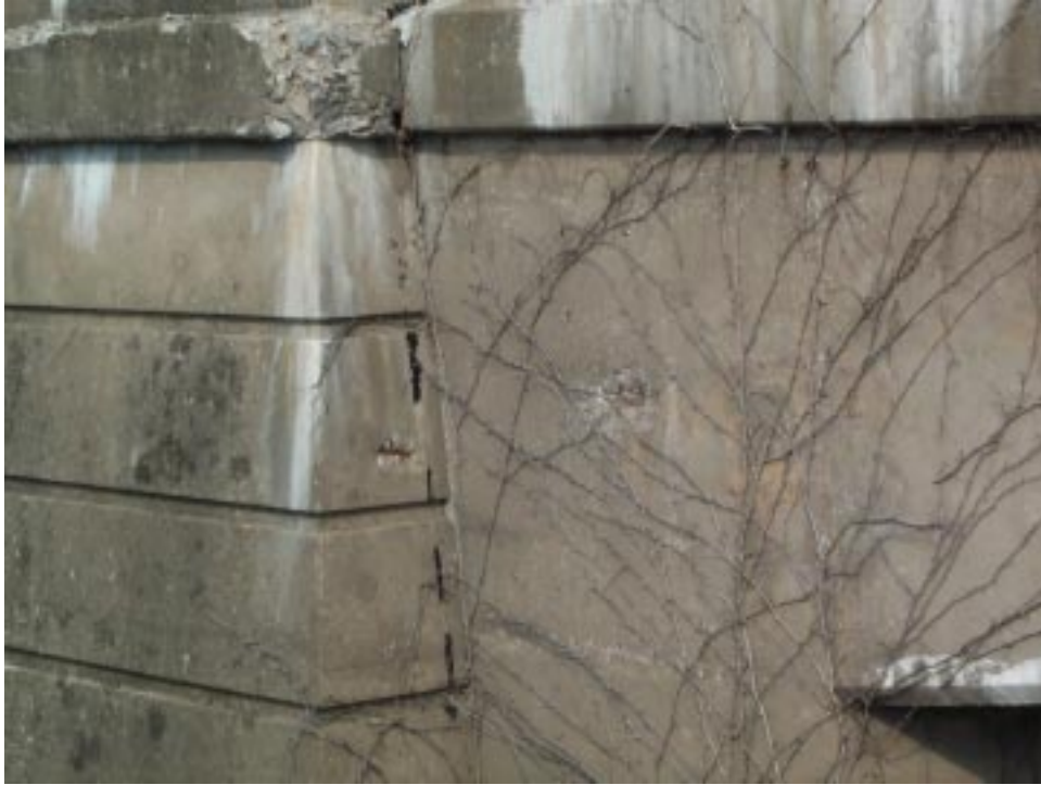
Figure 95. Inspector Photograph 9 – Localized spalling in northeast wingwall.
