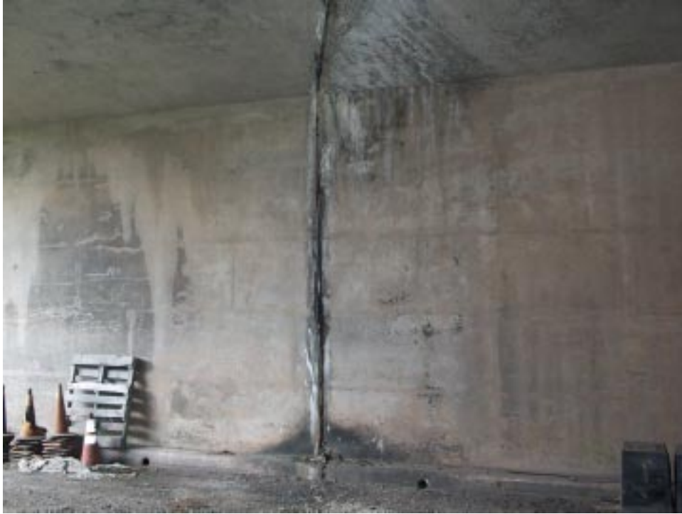
Figure 91. Inspector Photograph 5 – East backwall longitudinal joint deterioration.
