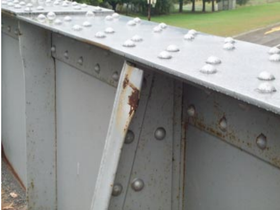
Figure 109. Deterioration described by Note A5 – Impact damage to superstructure stiffeners.
