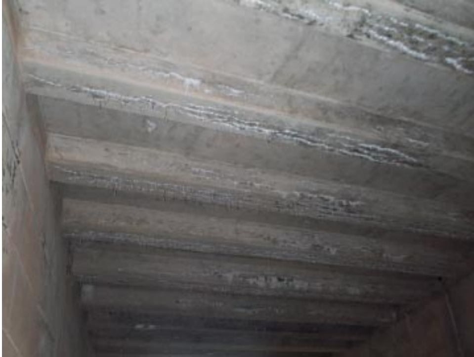
Figure 115. Deterioration described by Note C2 – T-beam deterioration.
