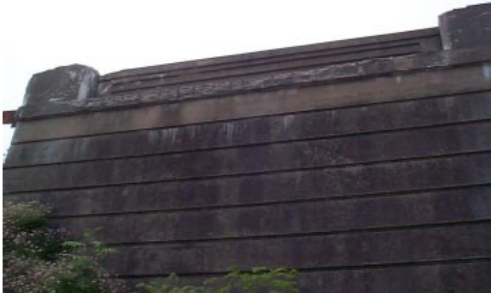
Figure 101. Inspector Photograph 15 – General wingwall condition.
