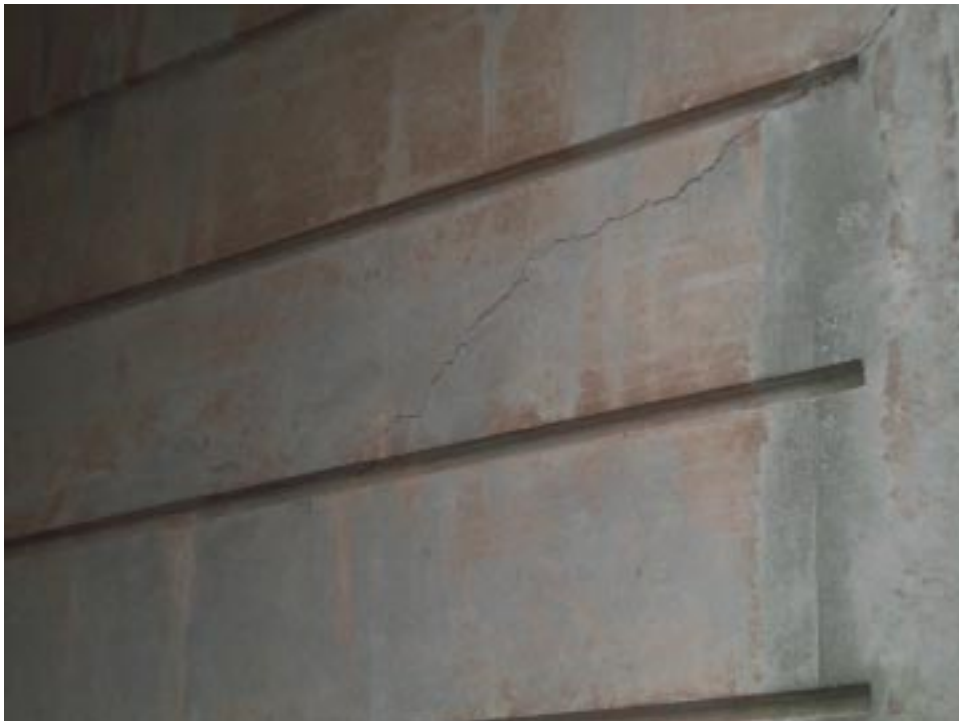
Figure 116. Deterioration described by Note C3 – Three-quarter length transverse crack in east abutment.
