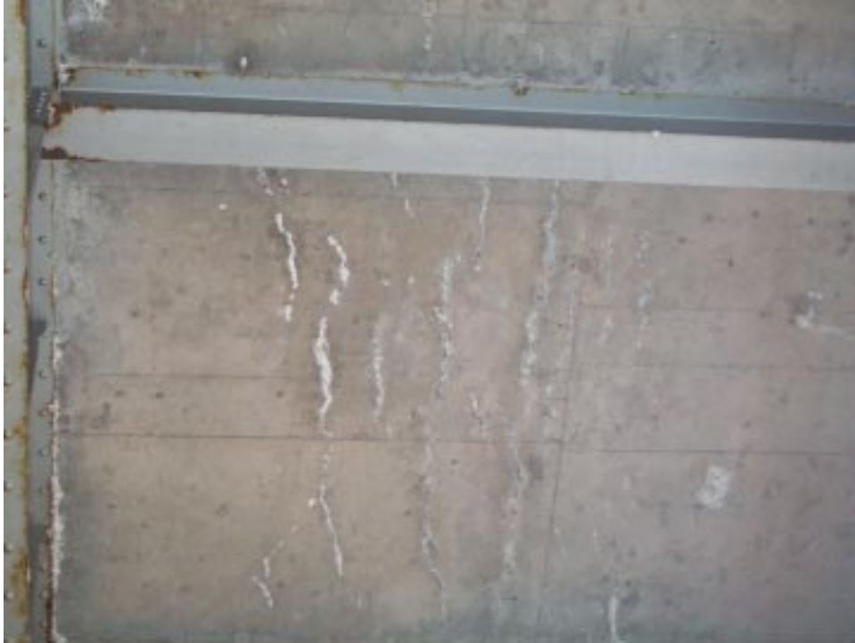
Figure 121. Deterioration described by Note E2 – Underside deck cracking and/or efflorescence.
