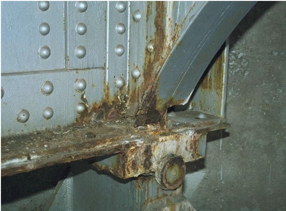
Figure 122. Deterioration described by Note E3 – Minor to moderate superstructure corrosion.
