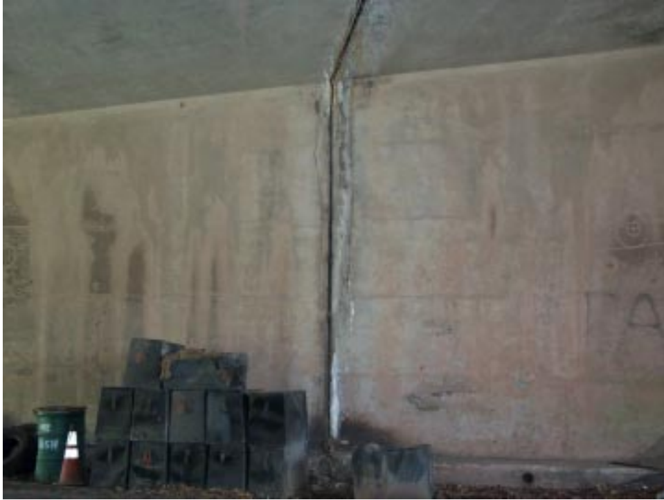
Figure 89. Inspector Photograph 3 – West backwall longitudinal joint deterioration.
