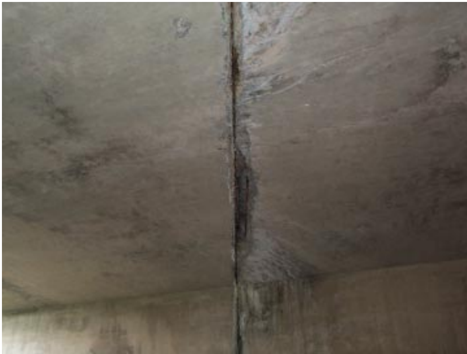
Figure 90. Inspector Photograph 4 – Underside deck longitudinal joint deterioration.
