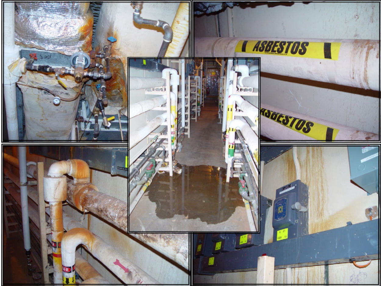
Photo 2. Maintenance problems at DX facilities.
