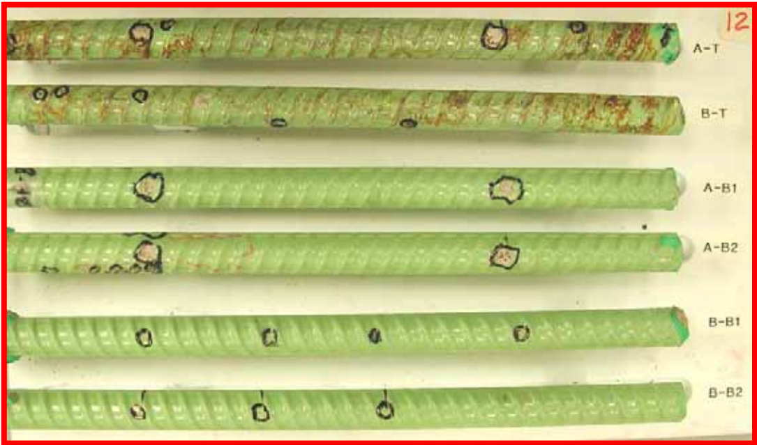
Figure 79. Slab #12 extracted rebars condition
