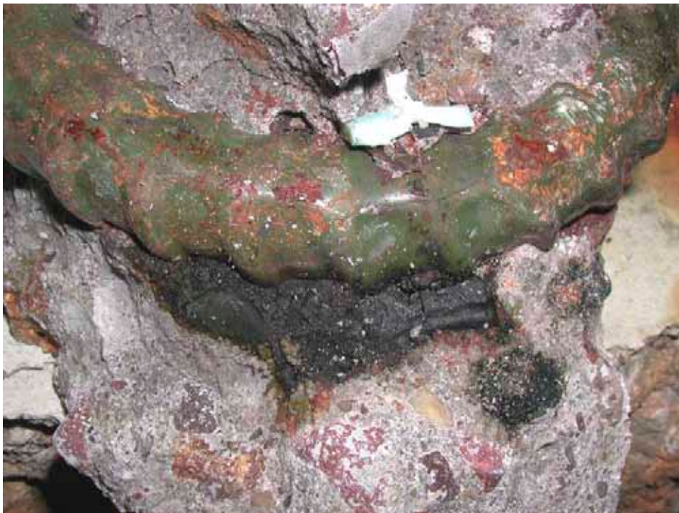
Figure 32. Typical condition of a bent ECR with poor performance
