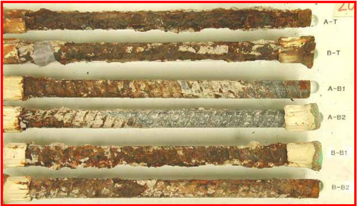
Figure 103. Slab #20 extracted rebars condition
