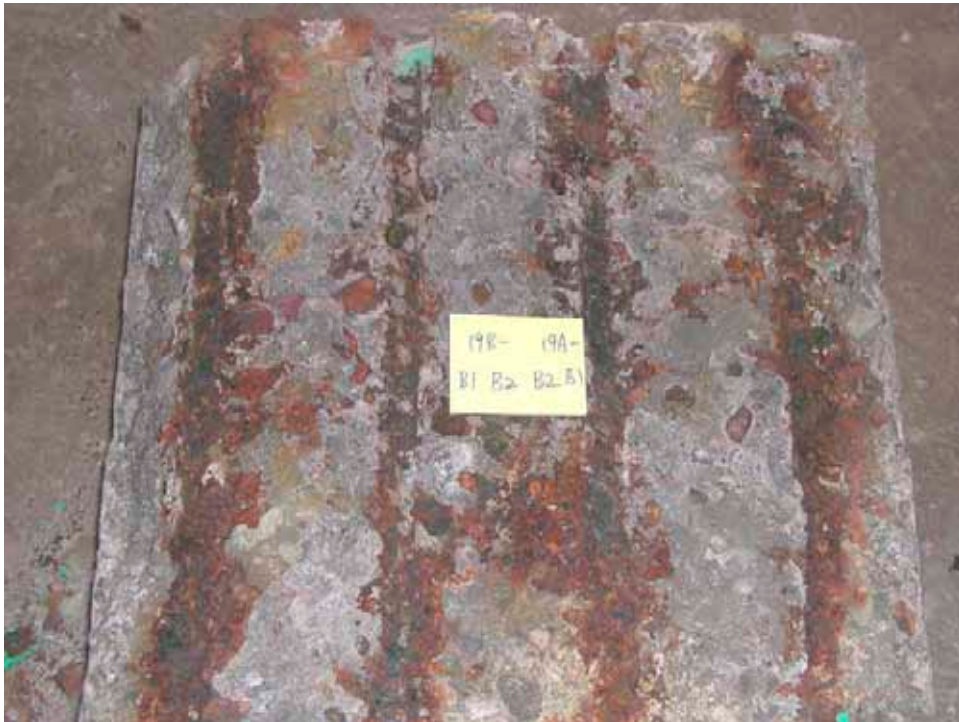
Figure 36. Corroded bottom mat (slab #19)
