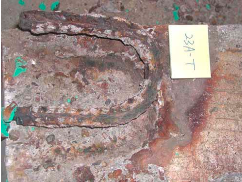
Figure 35. Typical condition of black bent bars in the top mat (slab #23—top right bar)
