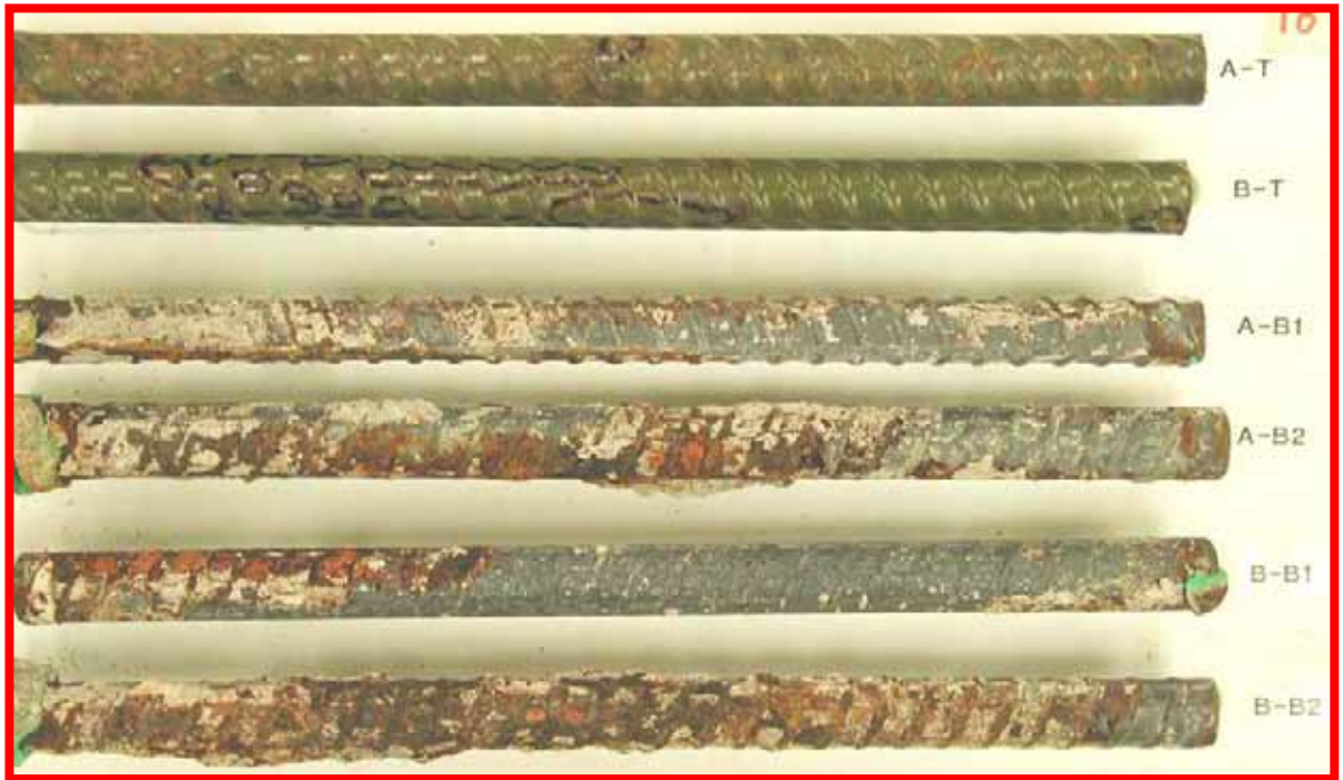
Figure 97. Slab #18 extracted rebar condition
