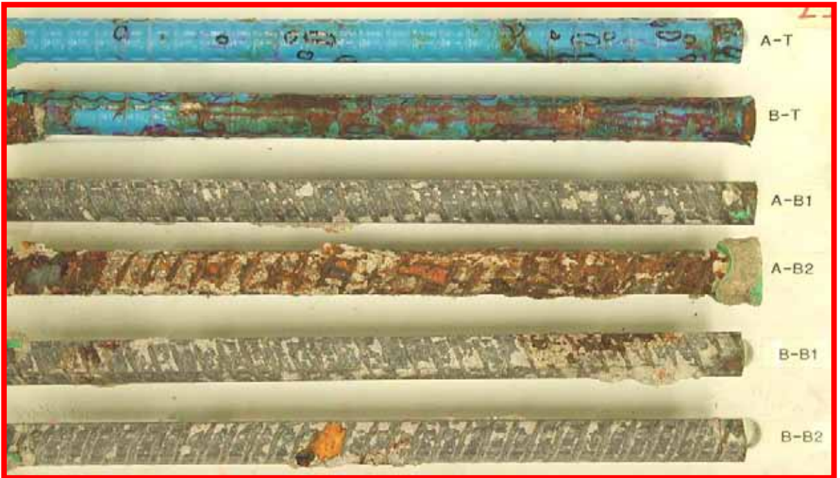
Figure 118. Slab #25 extracted rebar condition
