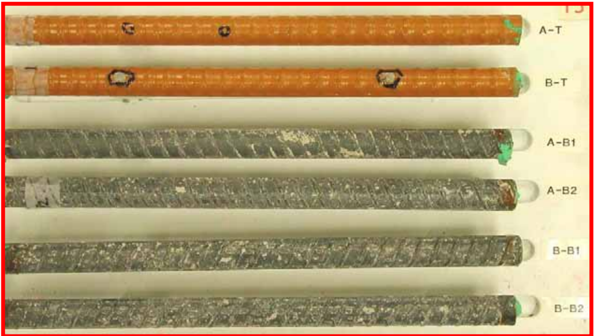
Figure 88. Slab #15 extracted rebar condition
