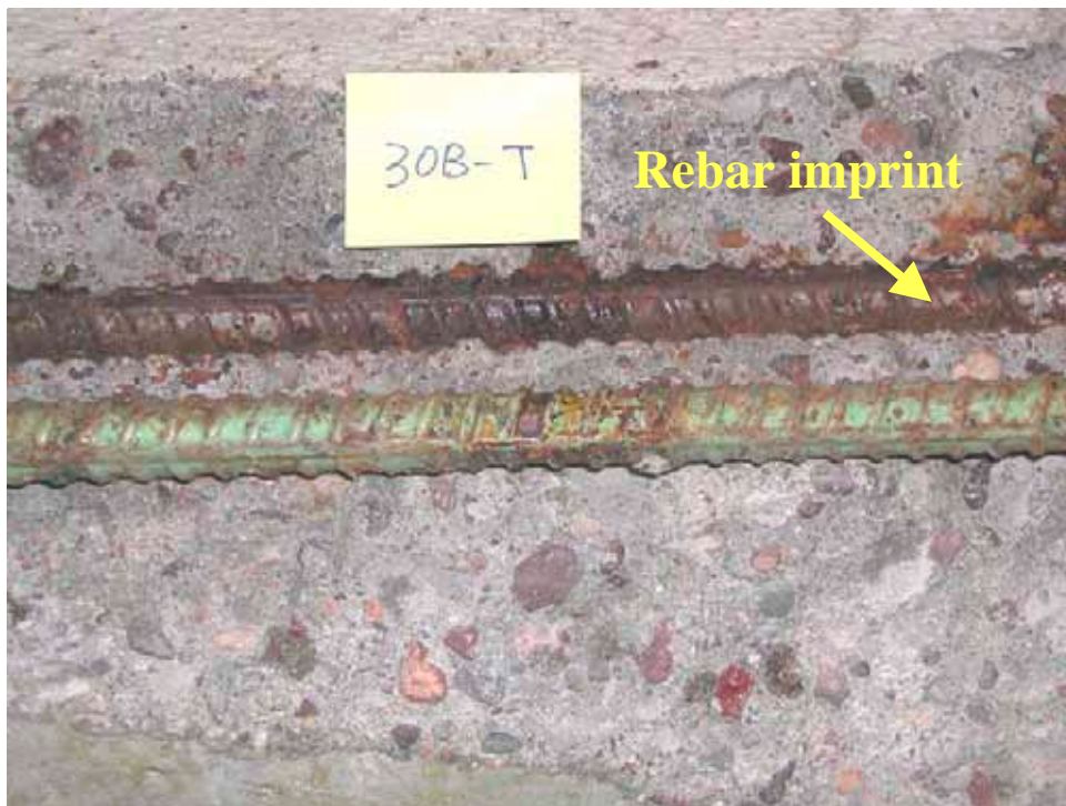
Figure 30. Typical condition of ECR with poor performance (slab #30—top right bar)
