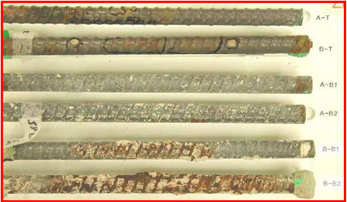
Figure 127. Slab #28 extracted rebars condition
