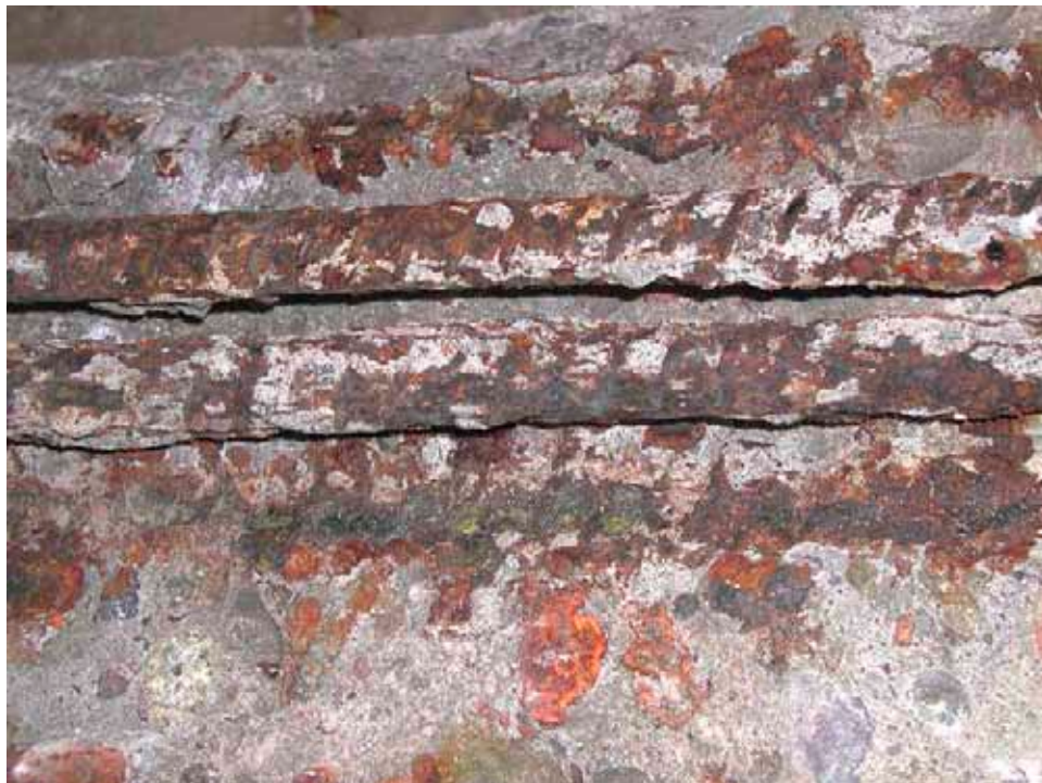
Figure 34. Typical condition of black bars in the top mat
