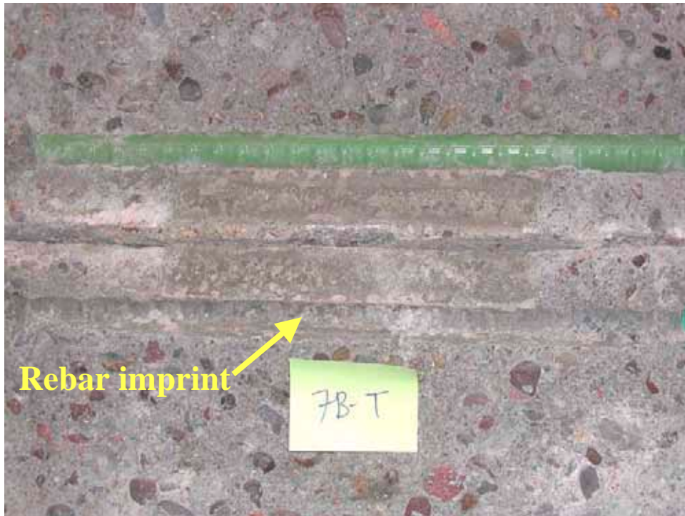
Figure 29. Typical condition of ECR with good corrosion resistance (slab #7—top right bar)
