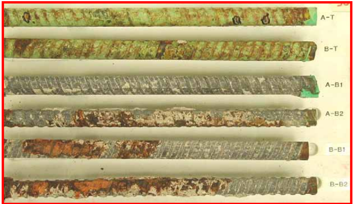
Figure 133. Slab #30 extracted rebars condition
