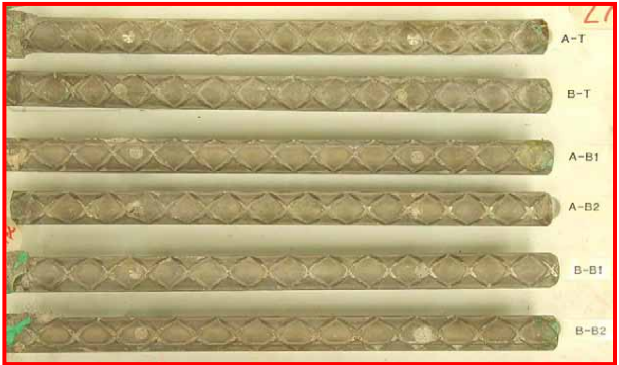
Figure 124. Slab #27 extracted rebars condition
