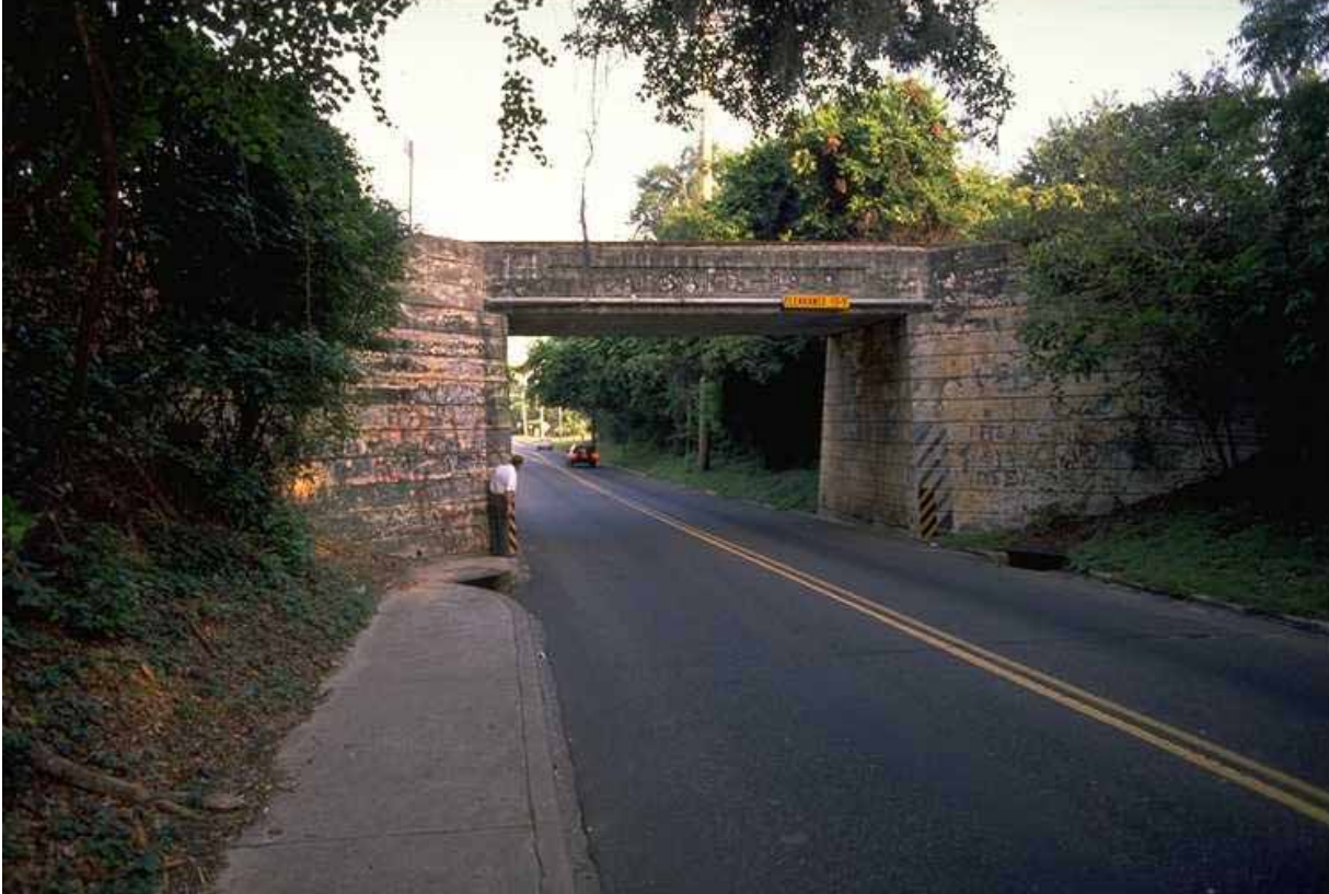
Figure 22-4. Photo. Example of a sidewalk ending at a bridge abutment with no warning or alternative path.
