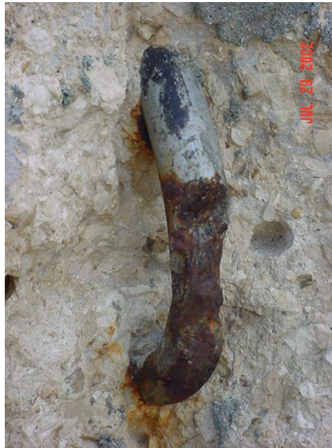
Figure 25. Corrosion of an exposed reinforcing bar.
