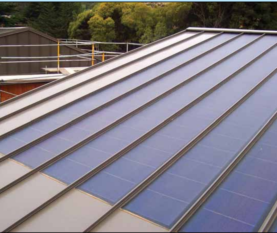
We are installing solar panels on the roofs of Fort Baker buildings to generate renewable energy.
