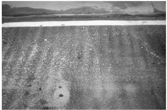
FIGURE 19-11 Washboard marks left by improperly operated vibratory roller.
