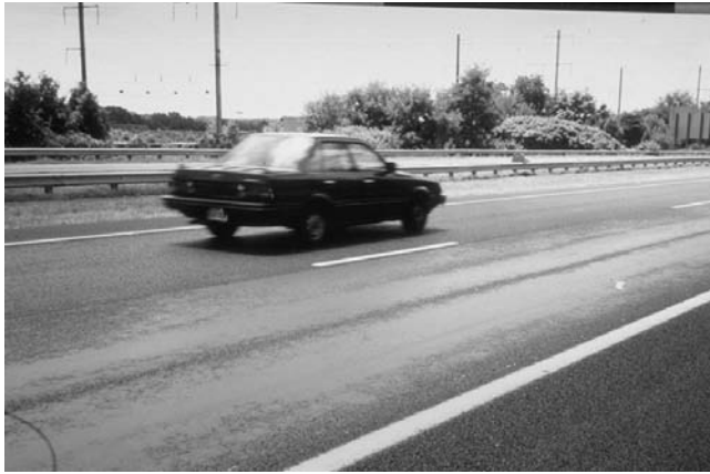
FIGURE 19-8 Fat spot caused by localized excess asphalt.
