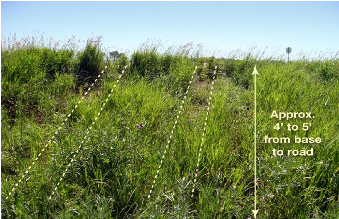
Dotted lines indicate where V2 entered embankment and the arrows show the approximate depth of the embankment.
