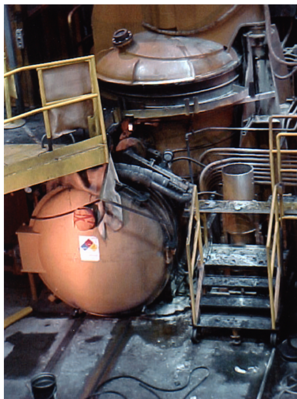
Exhibit #5. Skull Caster Furnace Showing Explosion Damage and NaK Residue
