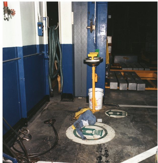
Exhibit #13. Safety Shower Showing Lack of Berms and Burned Clothing
