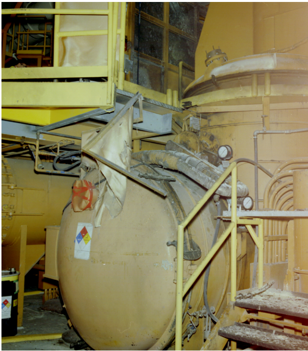
Exhibit #8. Furnace Showing Explosion Damage
