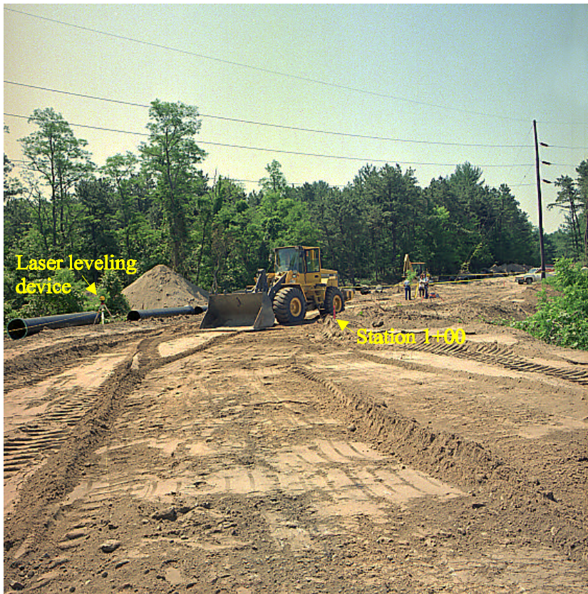
Exhibit 2-2. View of Accident Scene from Spoil Pile Facing South
