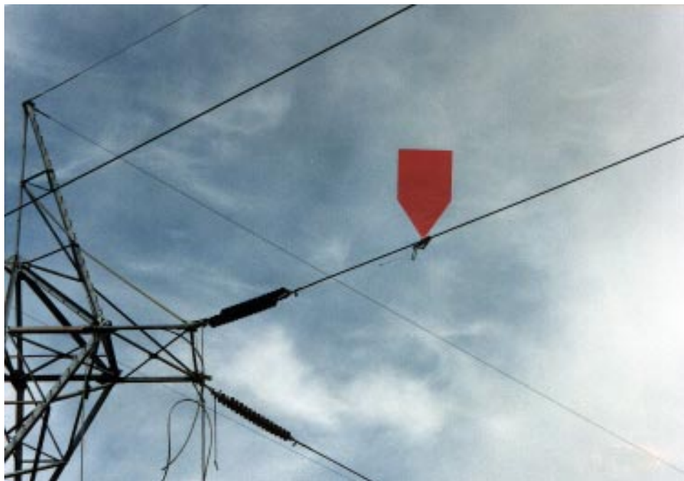
Exhibit 6 — Position of Grip on Conductor, Close-up.
