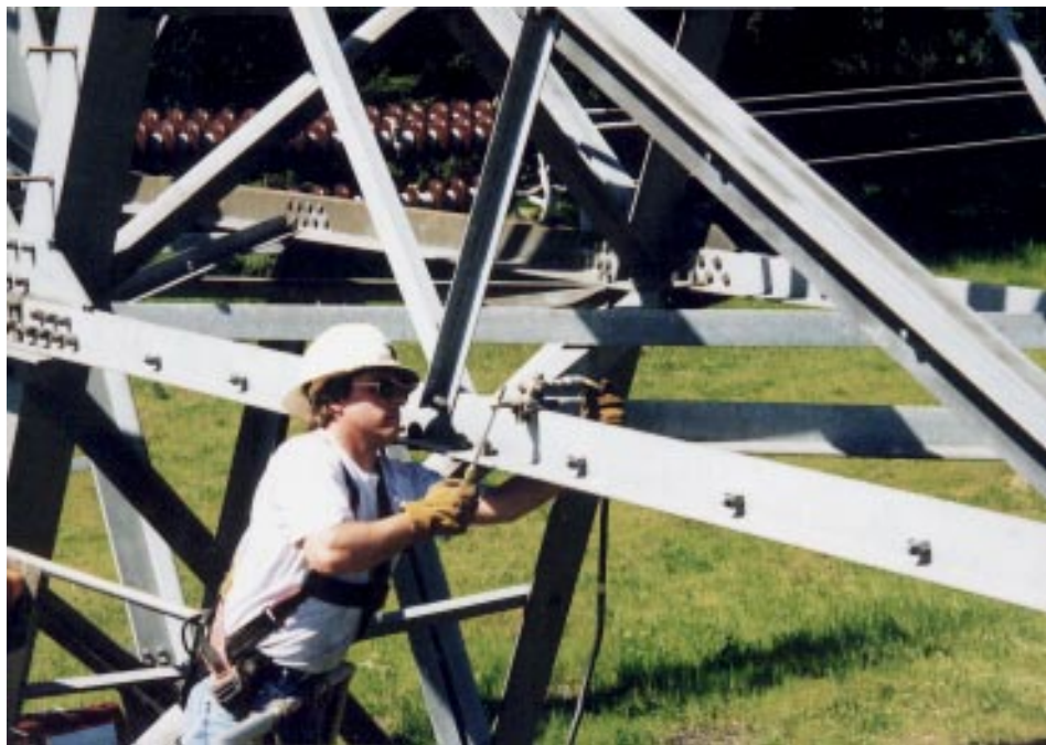
Photo B The worker is securing the ground end of the ground cable. It is important that a solid connection is made to ensure that a good electrical bond is achieved.
