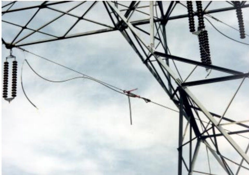
Exhibit 3 — Grip and Come-Along On Conductor at Scene of Accident
