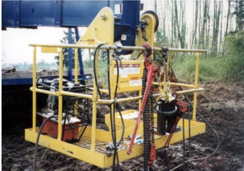
Exhibit 4 — Ungrounded Basket With Personal Ground Connections
