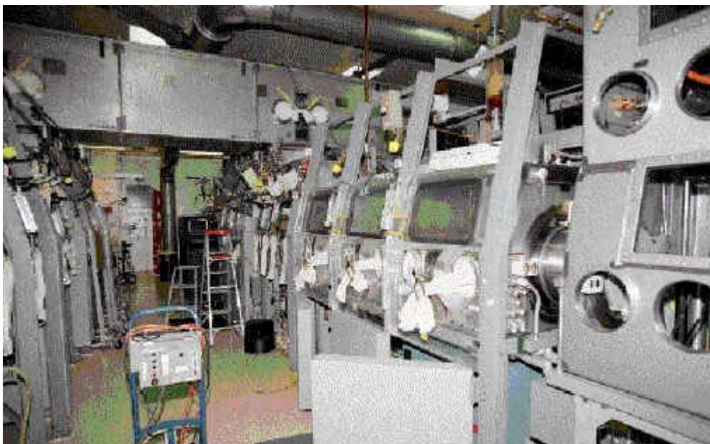
Exhibit 2-1. Affected Line of Gloveboxes
