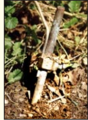
Grounding rod in the earth.
