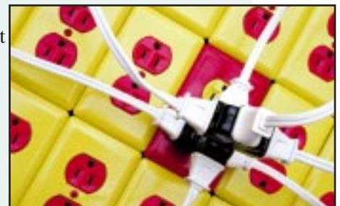
Overloads are a major cause of fires.
