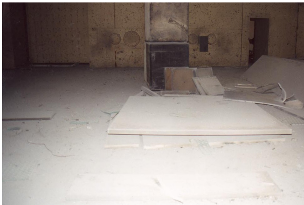
A Contained Firing Facility Chamber after an Explosive Test at LLNL
