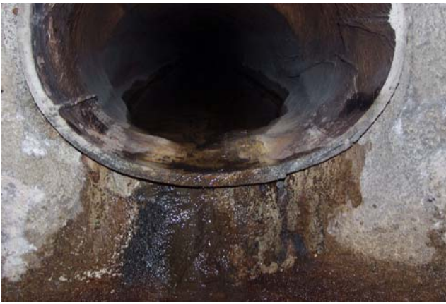
Lined Lateral Pipe
