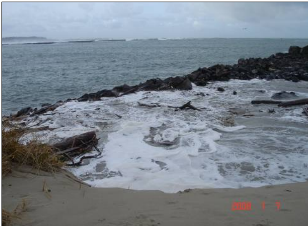
Figure 5. Repair Area 1, Active Jetty Overtopping at Stations 53+00 to 61+00
