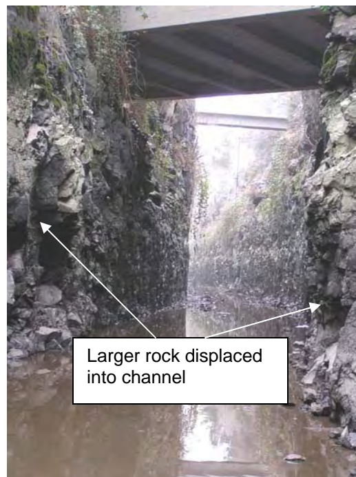
Photo G-2 Vertical slopes in the rock-lined channel. Notice zones where larger rocks have been displaced into channel. Only minor amount of rock debris on floor of the channel.
