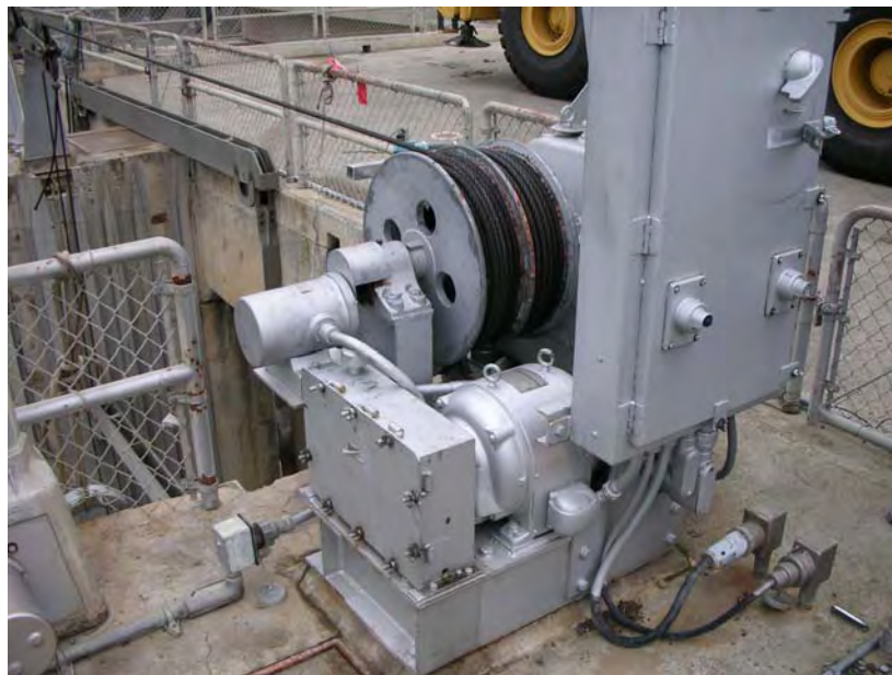
Photo ME-10 Hoists for raising and lowering telescopic gate at south fish entrance
