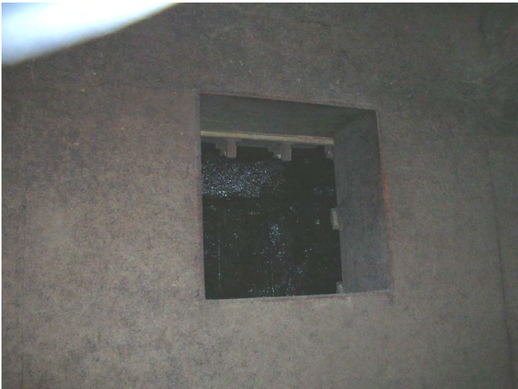
M-1 Diffuser Gate Opening In AWS Chamber
