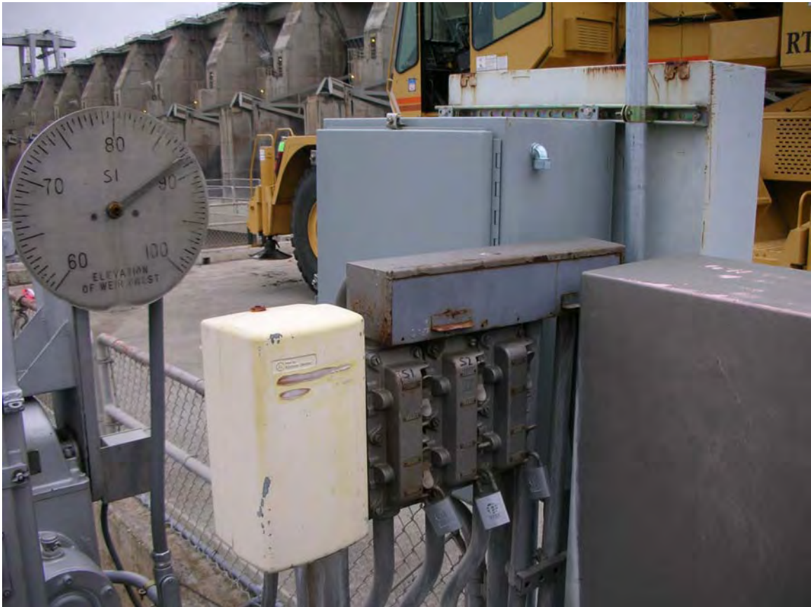
Photo ME-11 Hoist electrical controls at South Entrance showing older condition
