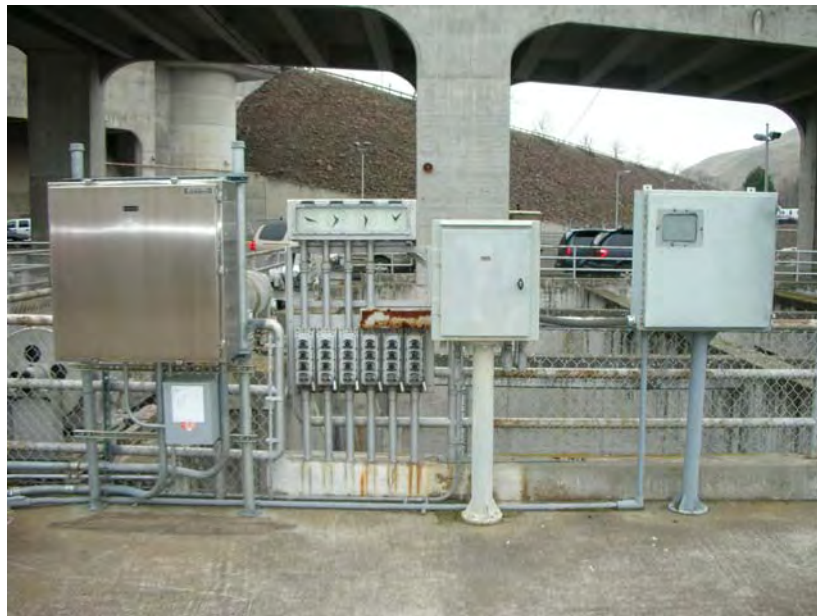
Photo ME-12 Hoist Control Station at Junction Pool
