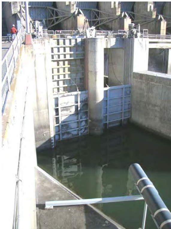
M-5 Entrance Weirs
