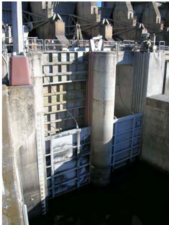
H-4 Entrance Weirs
