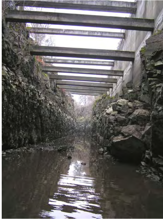
Photo G-3 – Area of rock-lined channel that is stabilized with concrete and cross struts.
