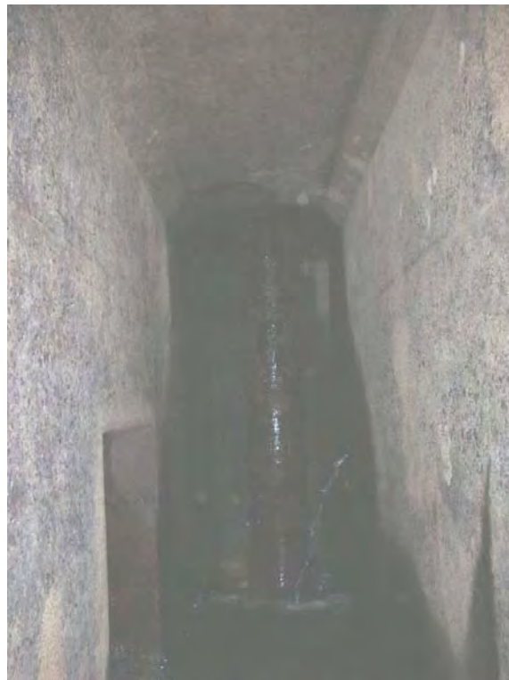
M-3 Conduit Dewatering Pump
