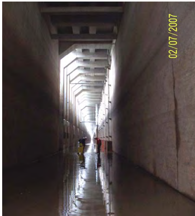
Photo H-5 Collection Channel
