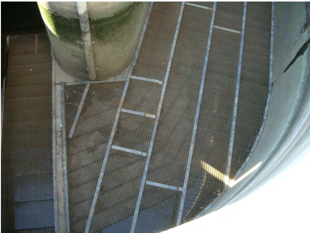
H-6 Entrance Pool Floor Diffuser Grating
