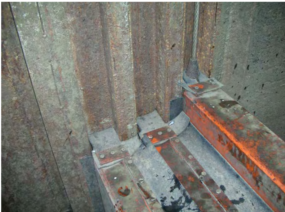
Photo ME-2 Leaf seals on the southernmost weir at East Entrance
