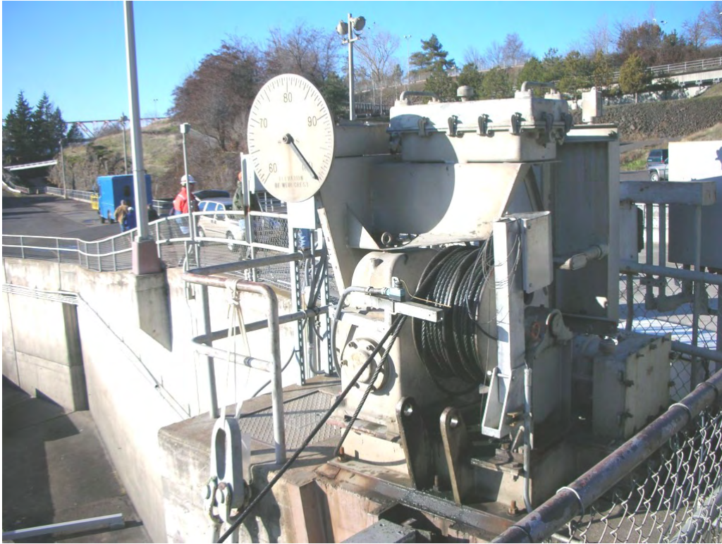
M-6 Entrance Weir Hoist For Gate N-1
