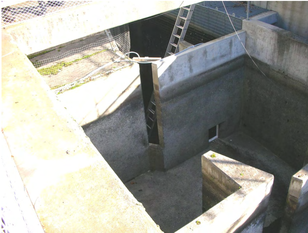
H-9 Exit Section Flow Control Weirs Looking Upstream
