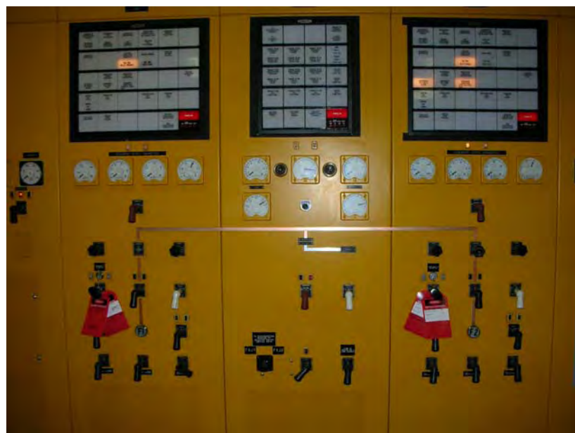
Photo ME-18 Fish Turbine Controls
