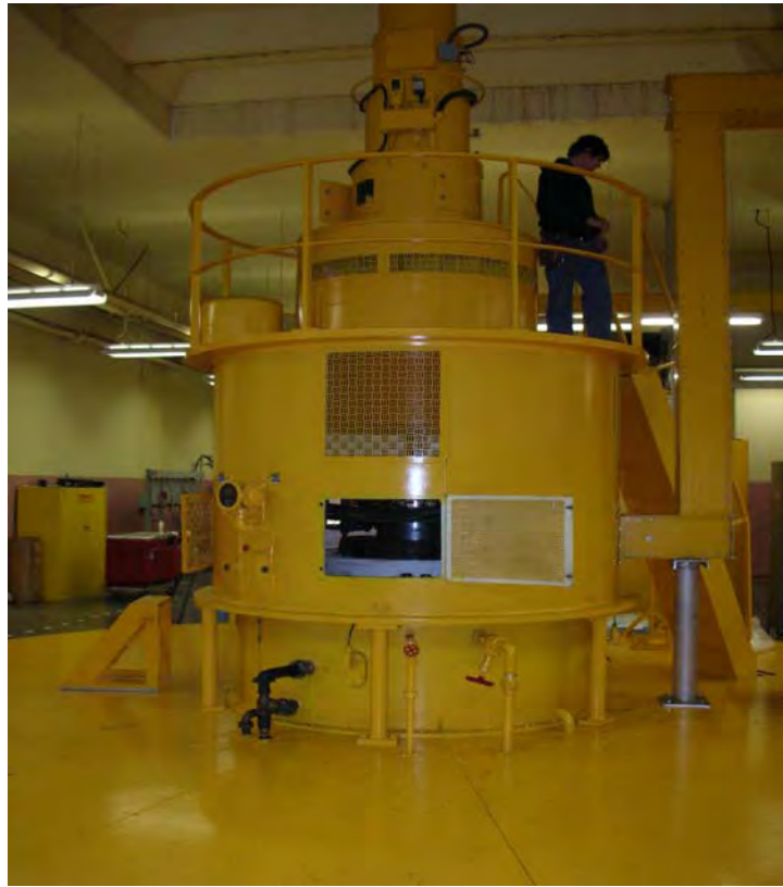
Photo ME-17 Fish Turbine Units
