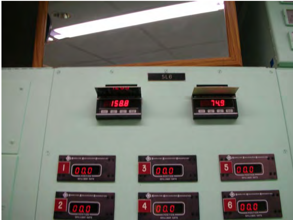
Photo ME-23 Fish Turbine Control Panels
