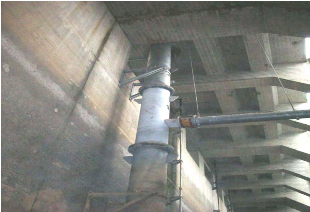
Photo ME-4 Dewatering pump casings along upstream side of collection channel
