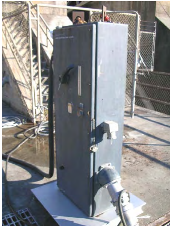
E-1 Dewatering Pump Panel
