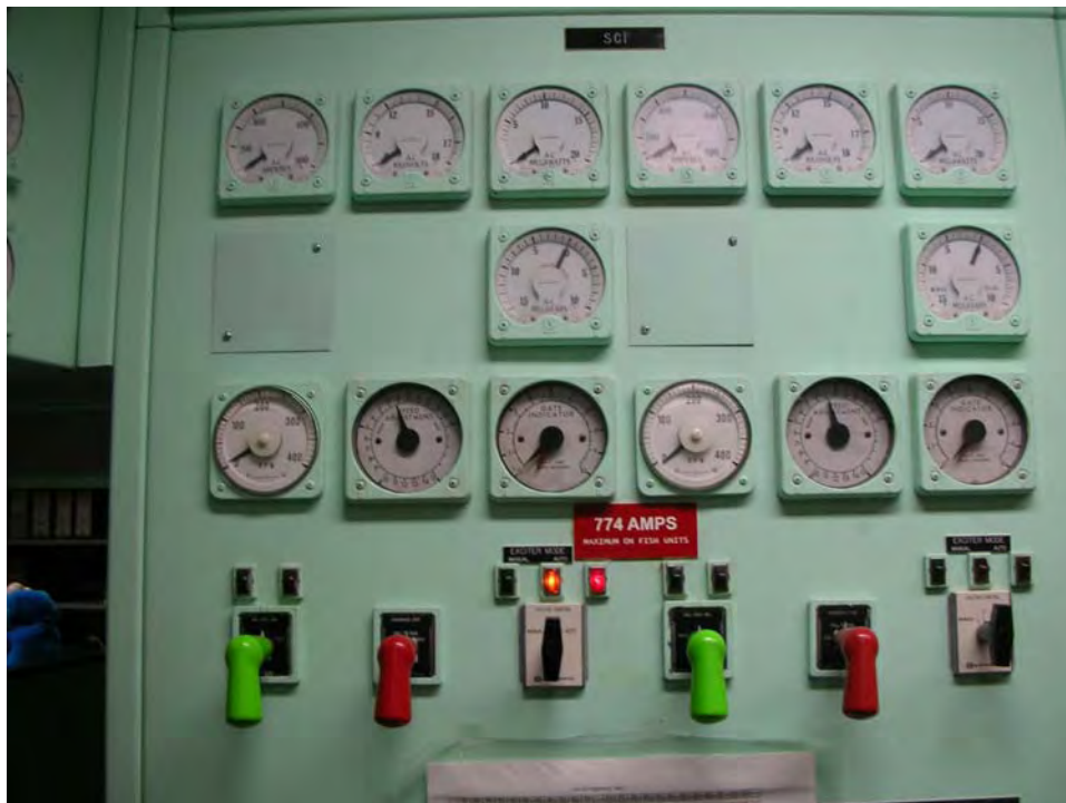
Photo ME-22 Fish Turbine Control Panels
