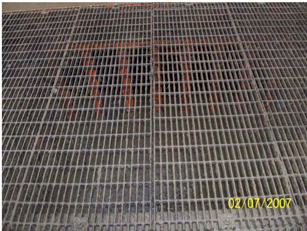
Photo H-8 Sediment on diffuser grating
