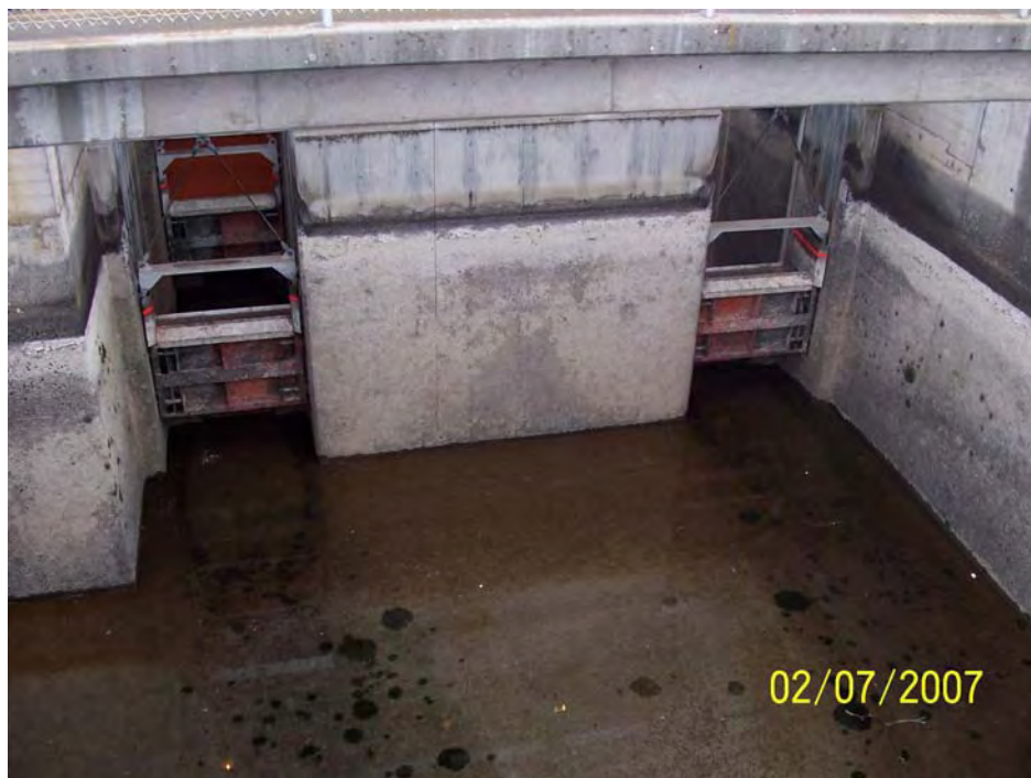
Photo H-14 Exit Weirs
