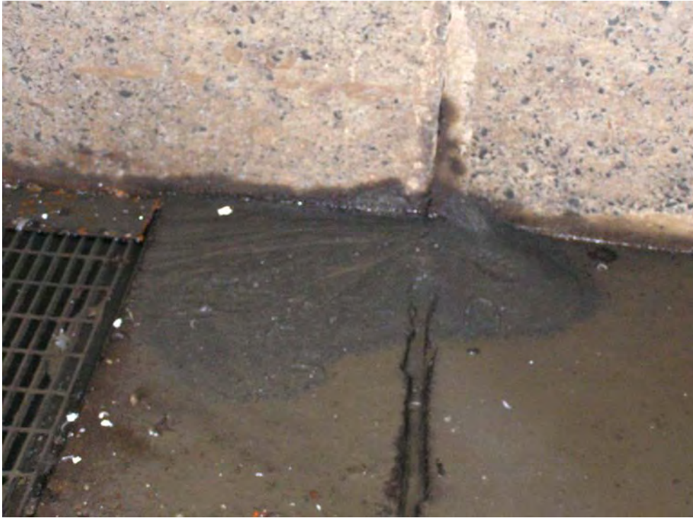
Photo CS-3 Sand accumulated from seepage at joint between concrete sections in Transportation Channel
