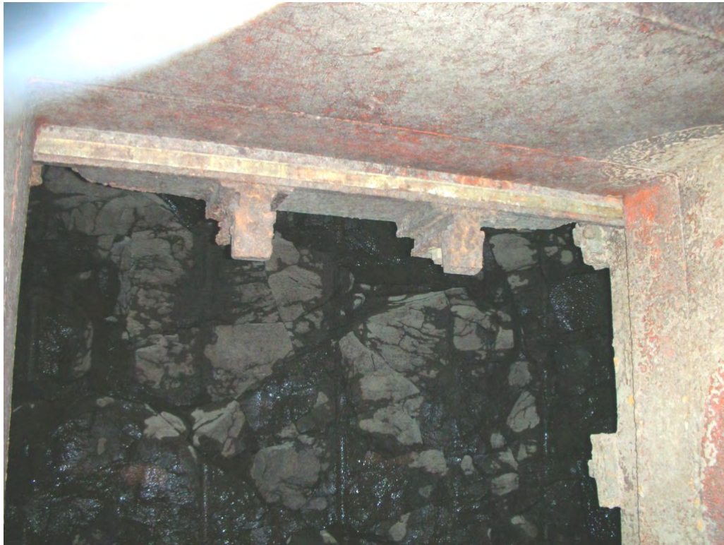
M-2 Diffuser Gate Corrosion
