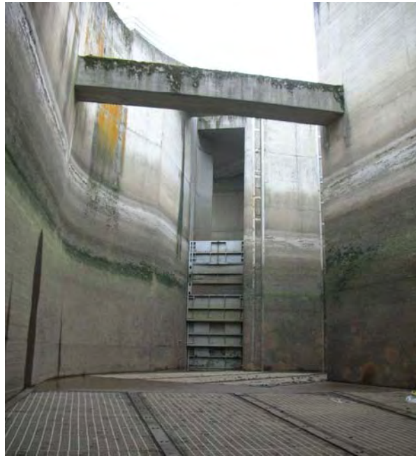
Photo ME-7 Telescoping “bypass” gate between collection and transportation channels
