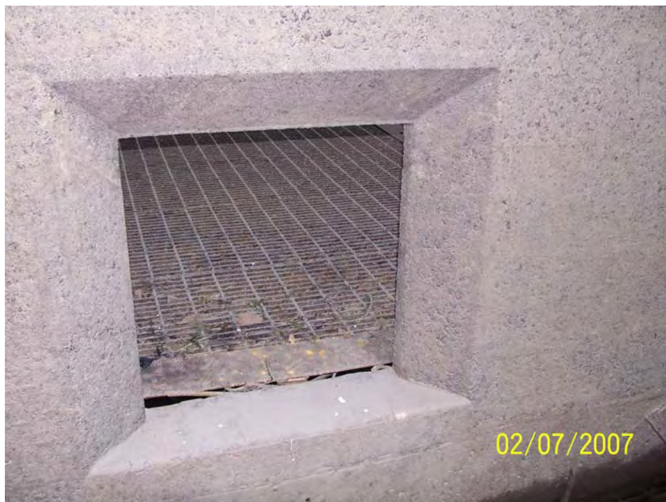
Photo H-4 Debris between diffuser grating and orifice
