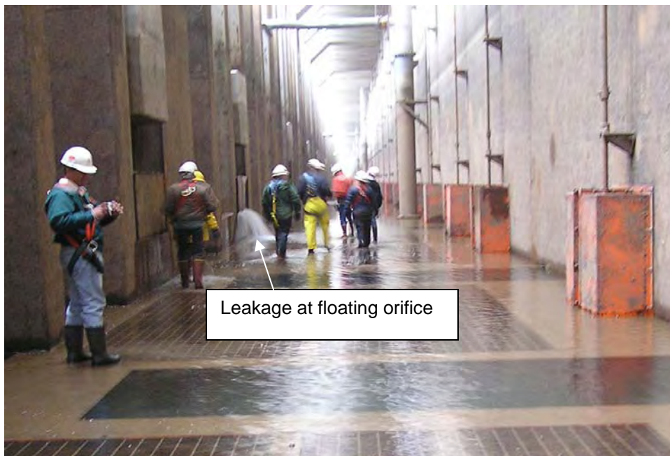
Photo CS- 2 Collection Channel. Note leakage at one floating orifice.
