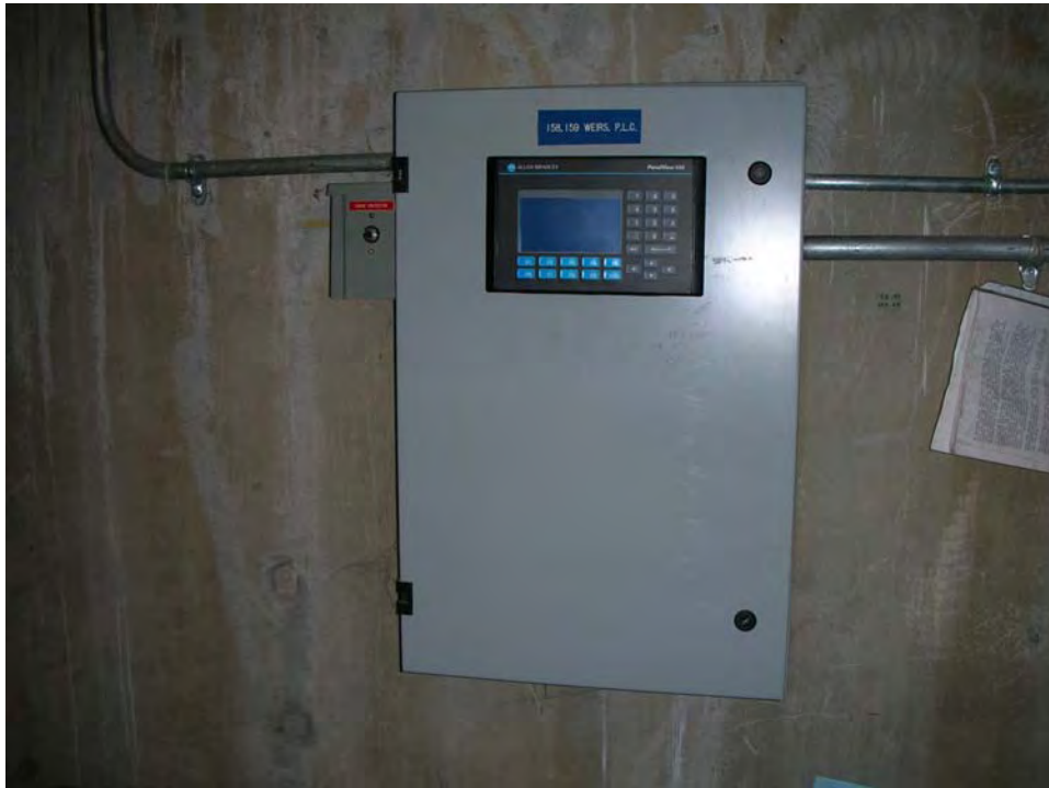
Photo ME-21 Motor Control Center and PLC
