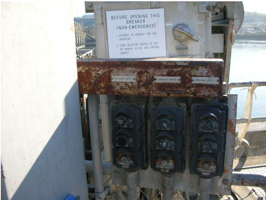
M-7 Entrance Weir Controls
