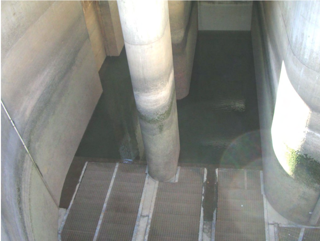
H-5 Entrance Pool Floor Diffuser Grating
