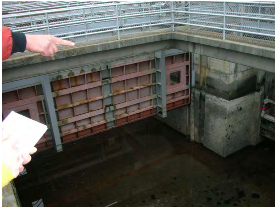
Photo ME-19 Adjustable weirs in fish ladder exit section
