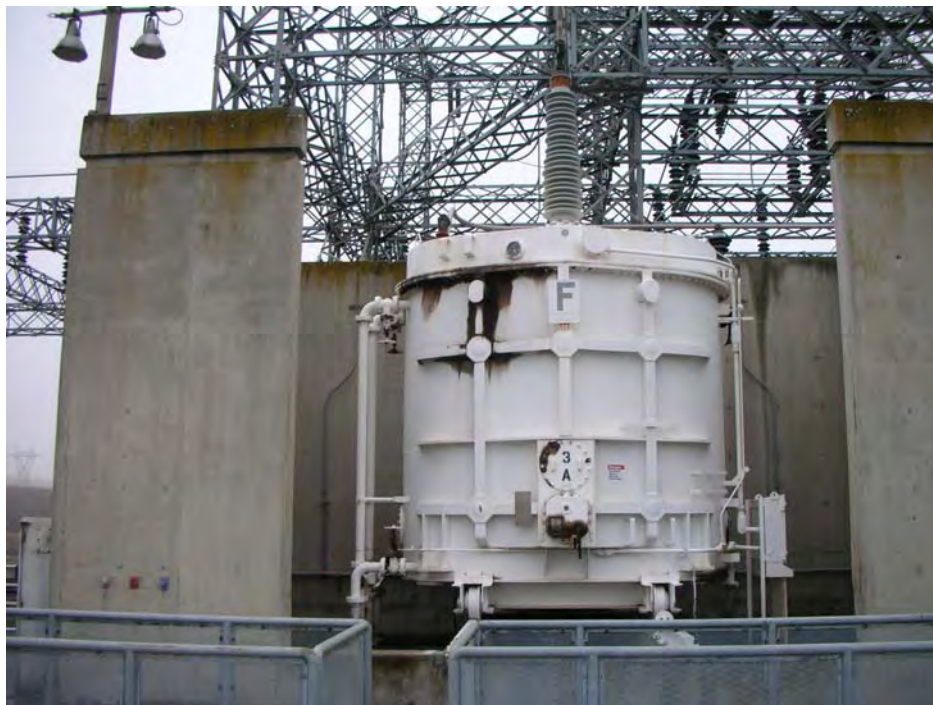
Photo ME-16 Fish Turbine Transformer
