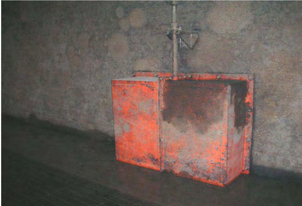
Photo ME-3 Diffuser gates along upstream wall of fish collection channel
