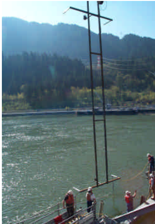
Figure 3. Installation of a 45-ft tall frame with split-beam transducers at the top and bottom center
