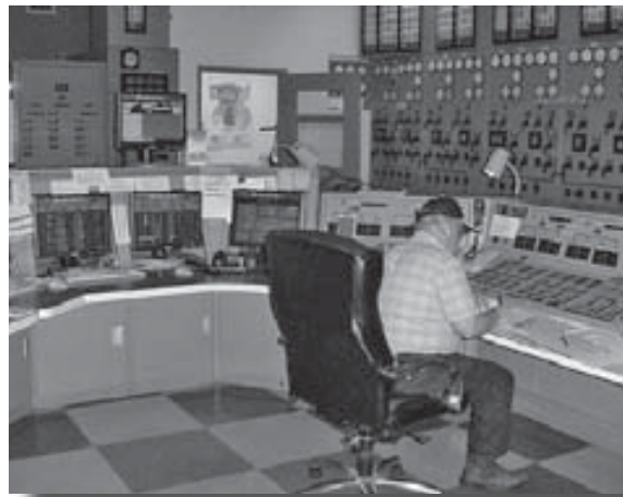
George Huff, senior chief operator at Chief Joseph Dam, mans the controls of the first dam to receive the T2 Optimization System software. The dam saved enough energy in 2007 to power more than 8,400 additional homes. Corps of Engineers Photo.
