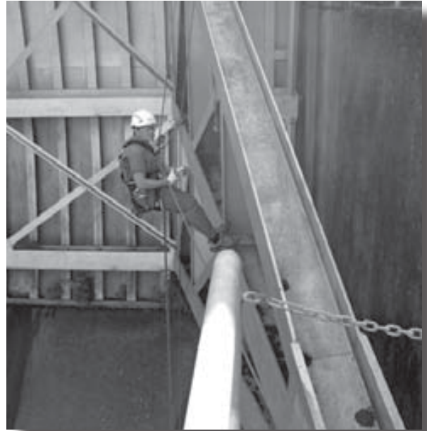
Climbers are lowered to inspect the steel struts, members and hinges on the Tainter gates at Foster Dam. Corps of Engineers Photo.
