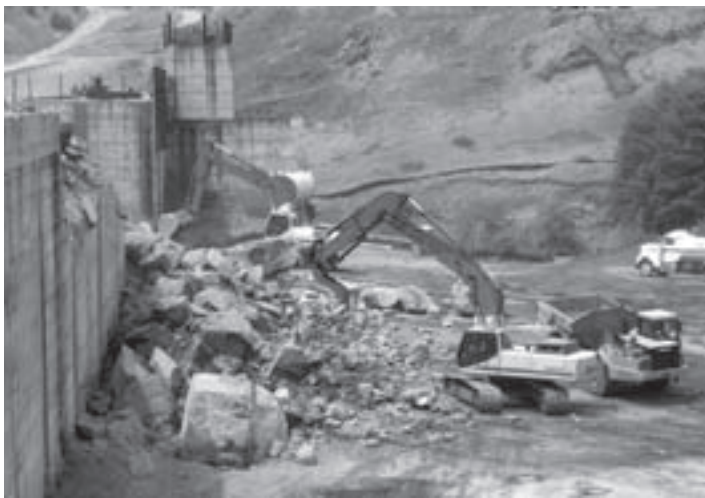
Despite the immense amount of debris generated by the blasting operations, workers took only seven weeks to create the entire notch through Elk Creek Dam.
