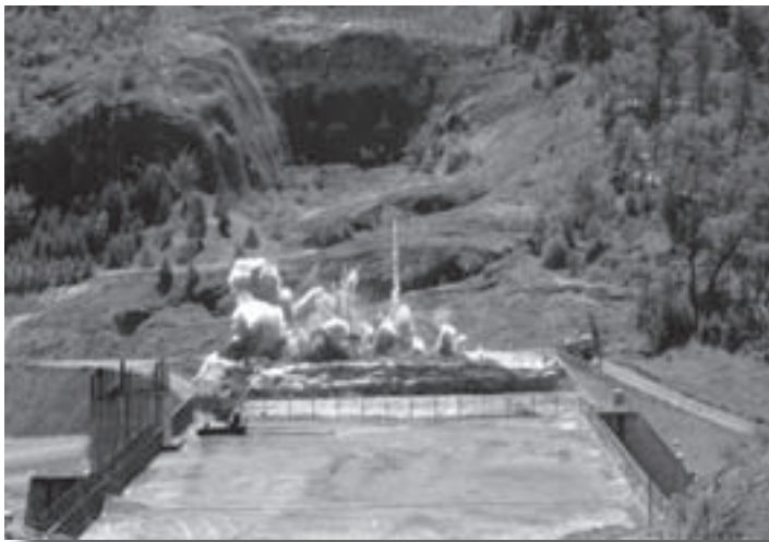
Fire in the hole! Demolition blast number three spanned the entire width of the left abutment and half its length.
