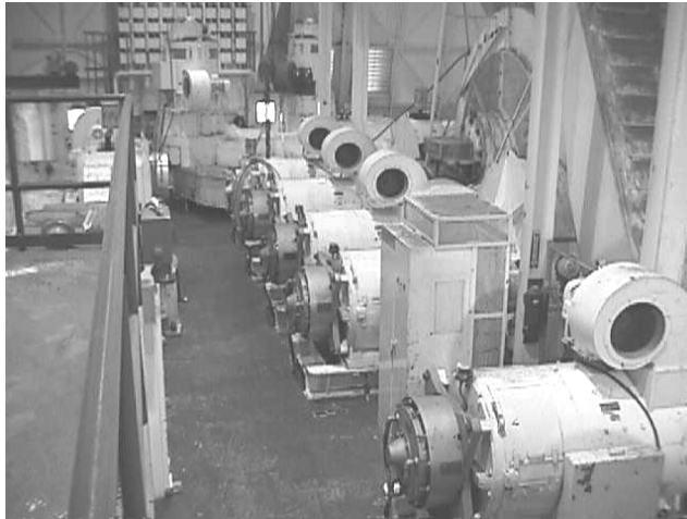
Figure 16.—Example of hoist and/or drag motors.
