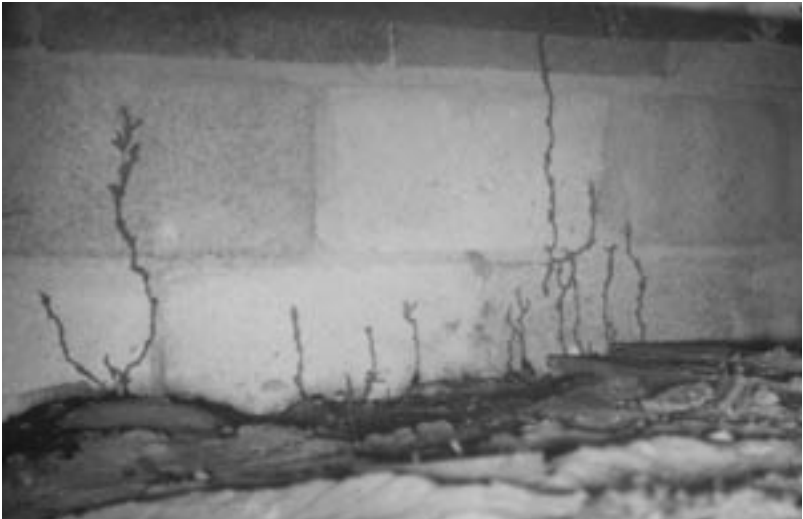
Figure 4. Termite tubes on the foundation of a structure.
