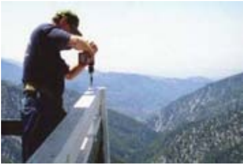
A volunteer provides much needed repair to the Butler Peak Lookout, bringing its rail hight to OSHA standards and ensuring the safety of over 7,500 visitors each year.
