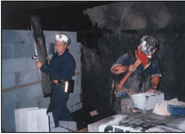
Installing load cells in a ventilation stopping in a longwall headgate to measure load development.
