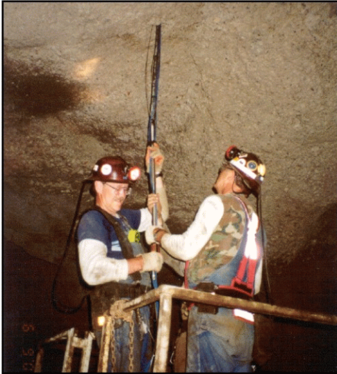
Project personnel install a 40-foot-long vertical borehole extensometer in cemented backfill to monitor displacement during mining beneath the backfill.
