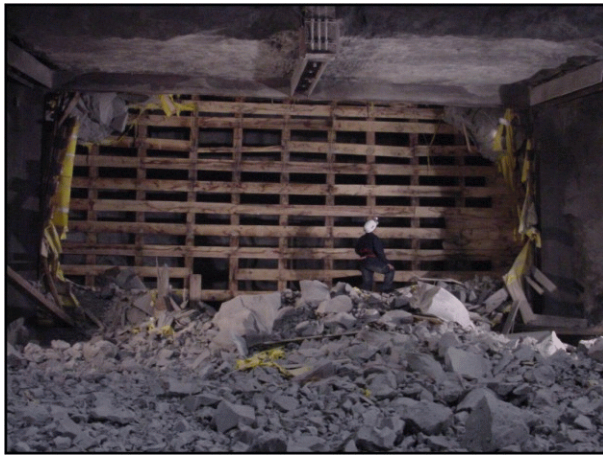
Remains of a cementitious seal after a methane air explosion.
