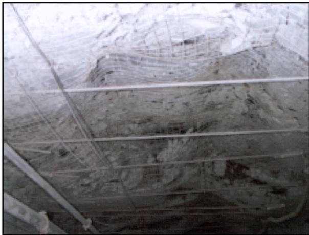
Anomalous deformation of the roof might indicate an impending roof fall.
