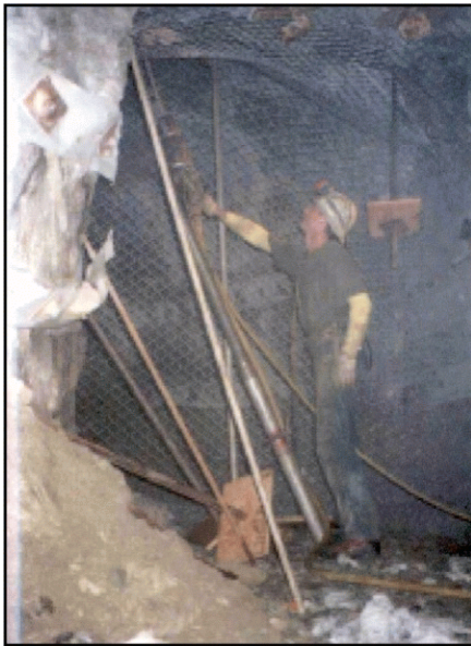
A new NIOSH video will demonstrate proper techniques for bolting roof rock safely.
