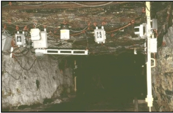
Mine fire sensor array in the Safety Research Coal Mine.
