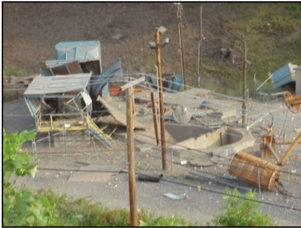
Shaft facility and fan house damaged by an underground mine explosion, Loveridge Mine, Marion County, WV. (Photo courtesy of MSHA.)
