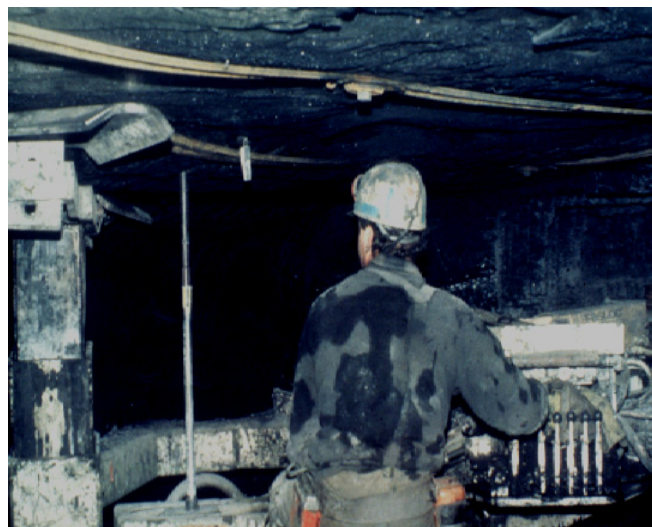
Figure 1.—The Analysis of Roof Bolt Systems (ARBS) helps select the proper roof bolt type and pattern.
