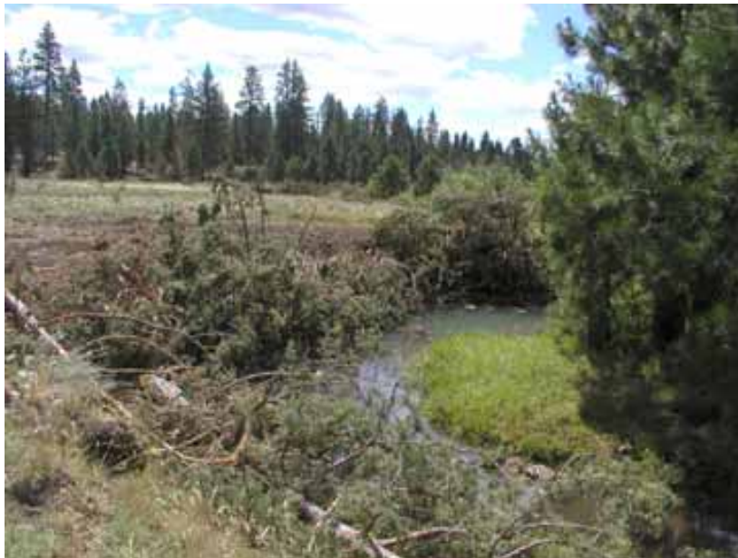
Same bank as above photo. Whole juniper trees used to armor bank.
