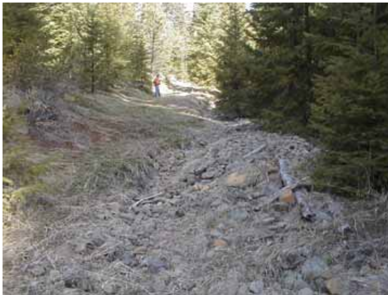
Erosion on Rd. 060.
