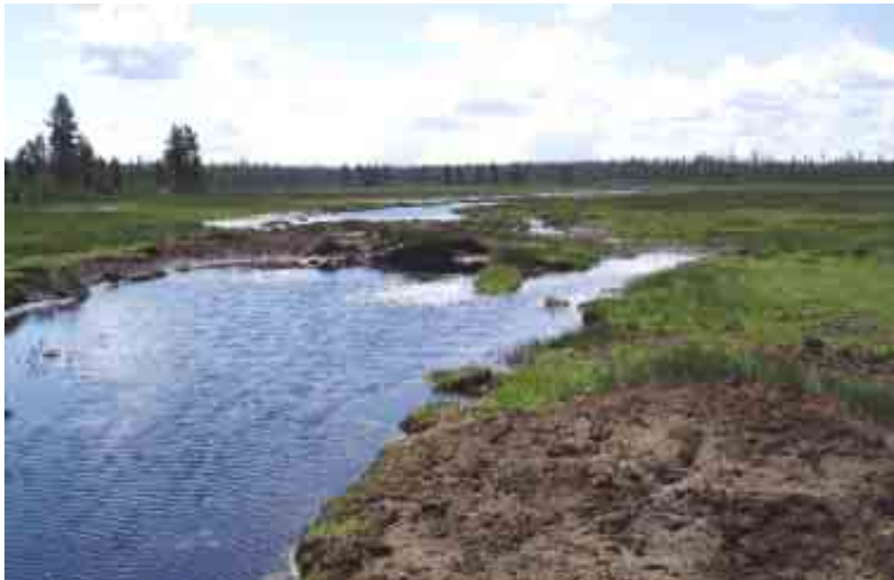
Photo 2: AFTER photo showing how a plug upstream of the crossing (30ft) is backing up the water and causing it to disperse to the left. At the lower end where the gradient increases there is some minor maintenance needed.
