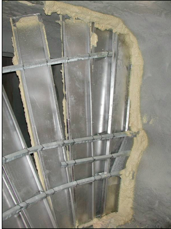
Figure 67.—Closeup of steel panel stopping still partially attached to outby rib in X-7 after LLEM test #458, viewed from B-drift.
