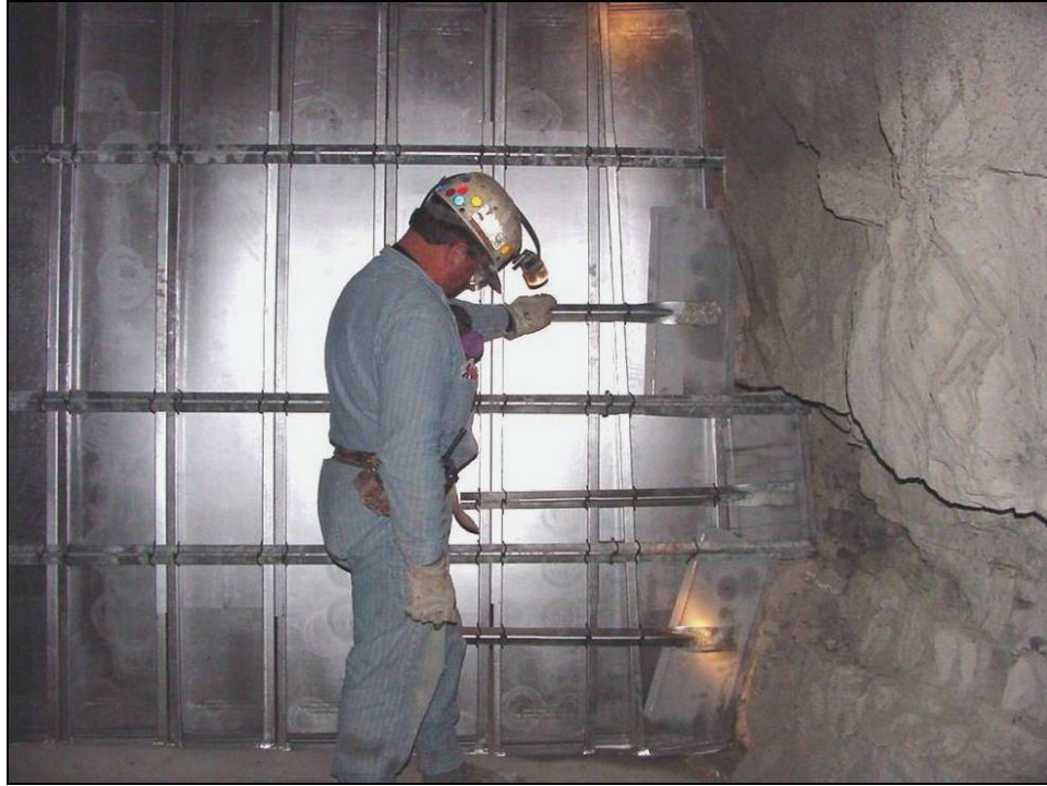
Figure 21.—Side extensions used to fill gaps between rib panel and rib, viewed from the back or B-drift side.
