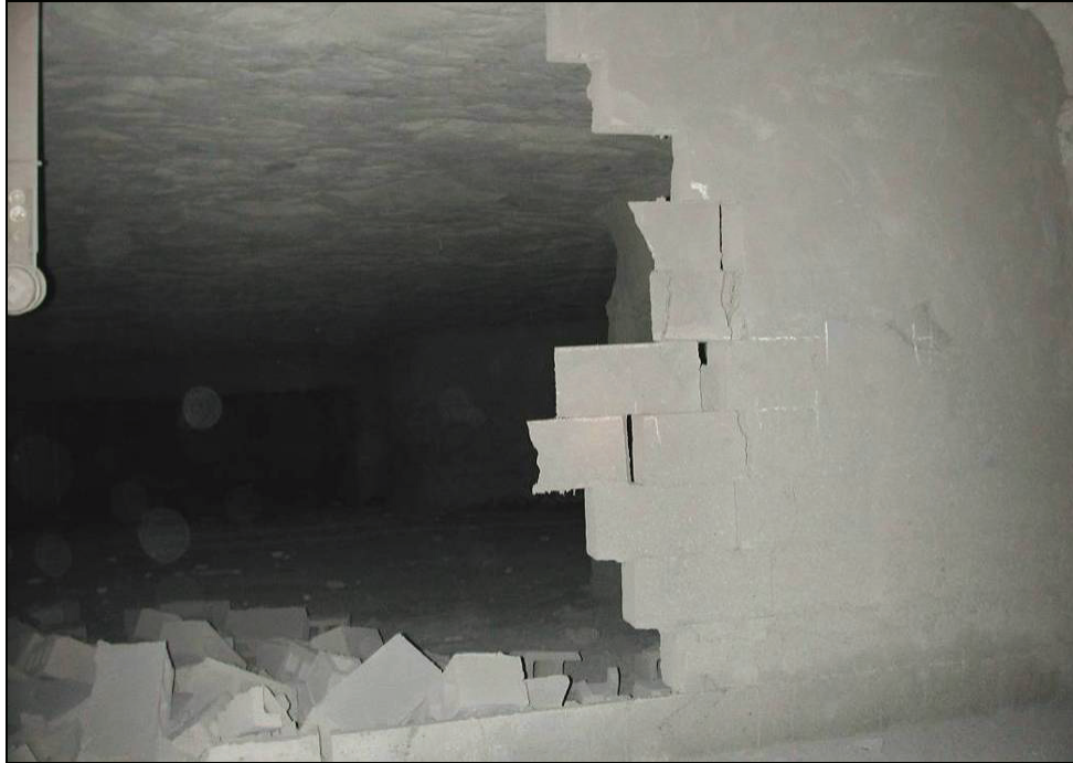
Figure 58.—Additional blocks partially dislodged from the right side of X-6 dry-stacked hollow-core concrete block stopping after test #434, viewed from C-drift.
