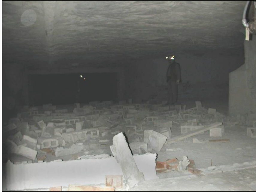
Figure 34.—Debris from dry-stacked hollow-core concrete block stopping in X-4 after LLEM test #428, viewed from C-drift.
