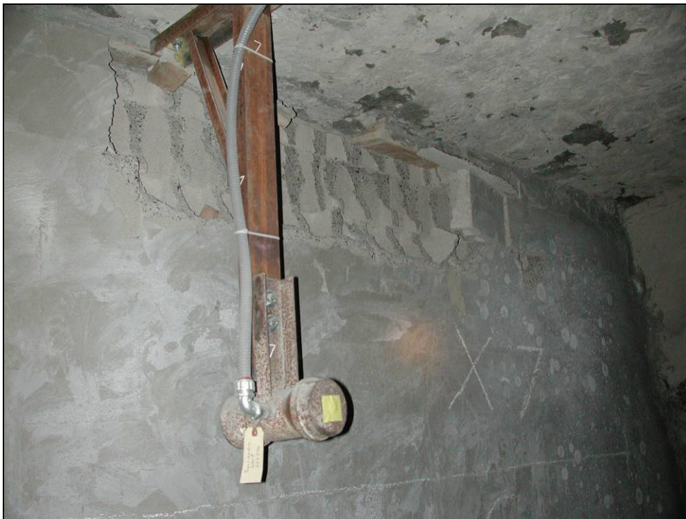
Figure 55.—Expanded view of top part of X-7 dry-stacked hollow-core concrete block stopping after explosion test #433, showing damaged blocks.
