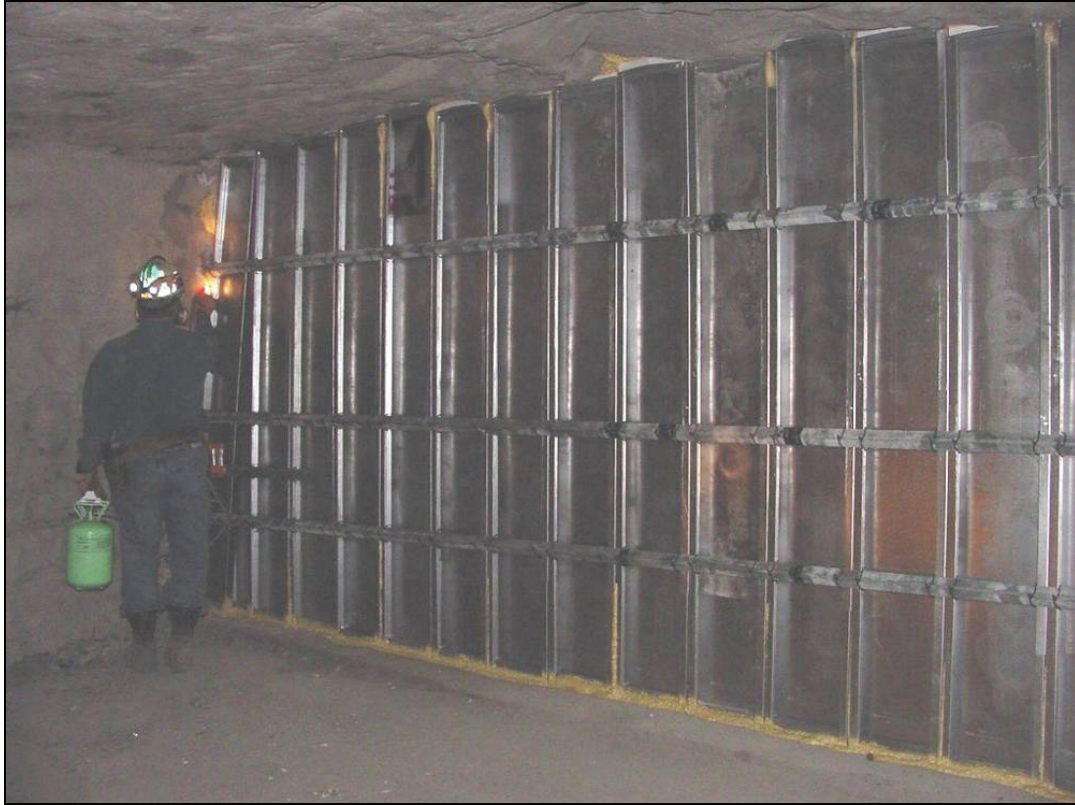
Figure 24.—Nearly completed steel panel stopping in X-6 showing the open panel side attached to the horizontal rib-to-rib angles on the B-drift side.
