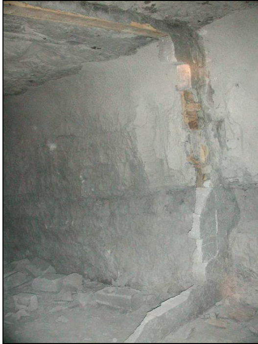
Figure 73.—Debris from the dry-stacked solid-concrete-block stopping and remaining blocks on the inby rib line in X-4 after LLEM test #462, viewed from C-drift.
