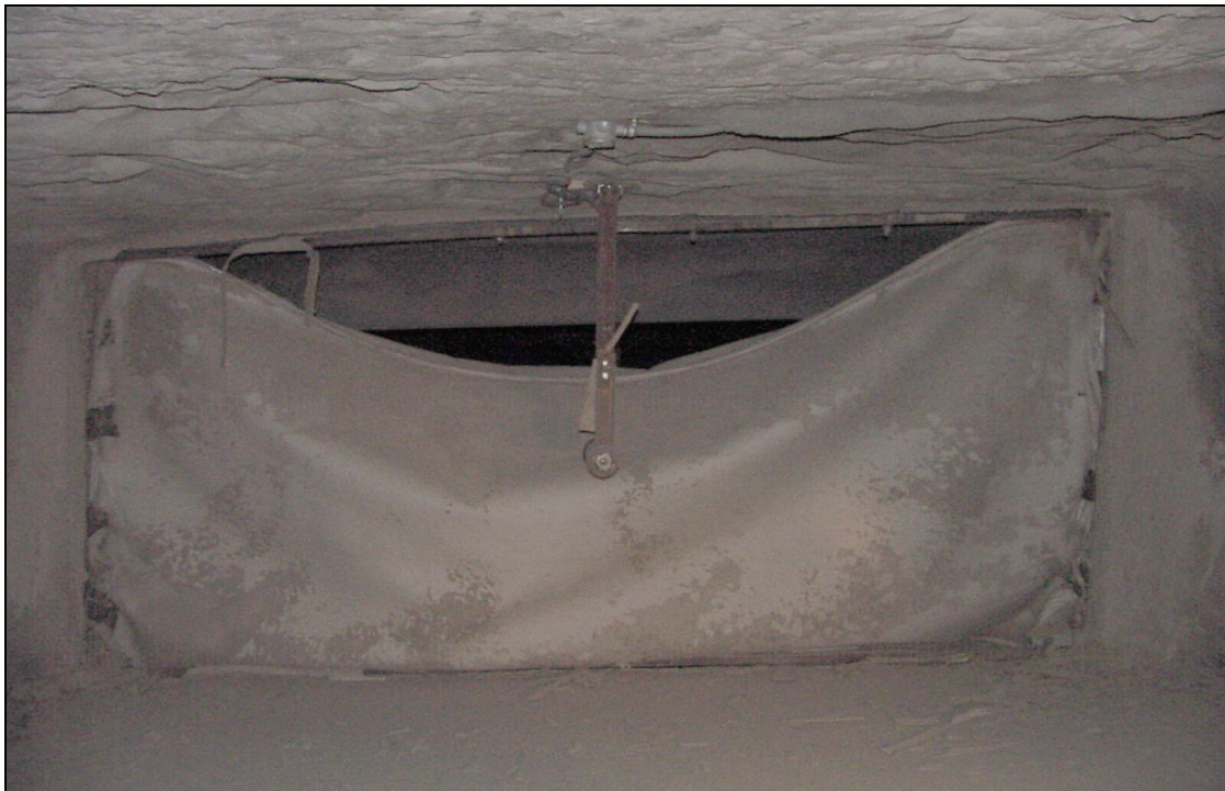
Figure 106.—Damage to the woven cloth stopping in X-7 after LLEM test #462.
