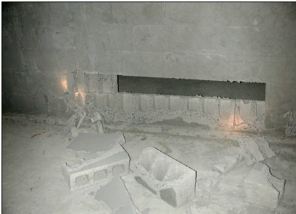
Figure 46.—Closeup of B-drift side of X-6 dry-stacked hollow-core concrete block stopping after test #430, showing dislodged and damaged blocks. This is clear evidence of roof-to-floor arching action.
