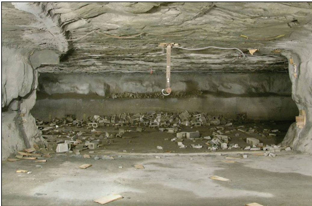
Figure 92.—Debris from the X-4 dry-stacked hollow-core concrete block stopping between A- and B-drifts after LLEM test #497.
