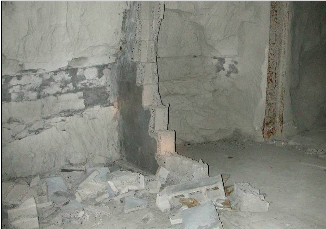
Figure 39.—Remnants of the dry-stacked hollow-core concrete block stopping in X-5 after LLEM test #428. The block shearing indicates roof-to-floor arching action.
