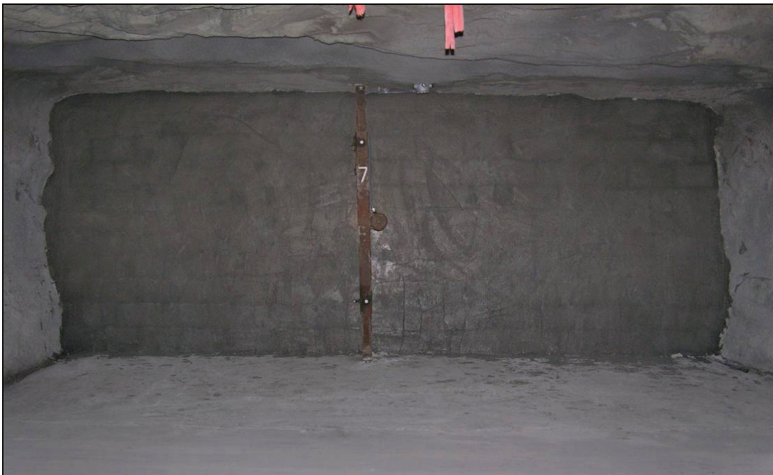
Figure 13.—Completed 6-in (15-cm) thick, wet-laid solid-concrete-block stopping in X-7, as viewed from A-drift.
