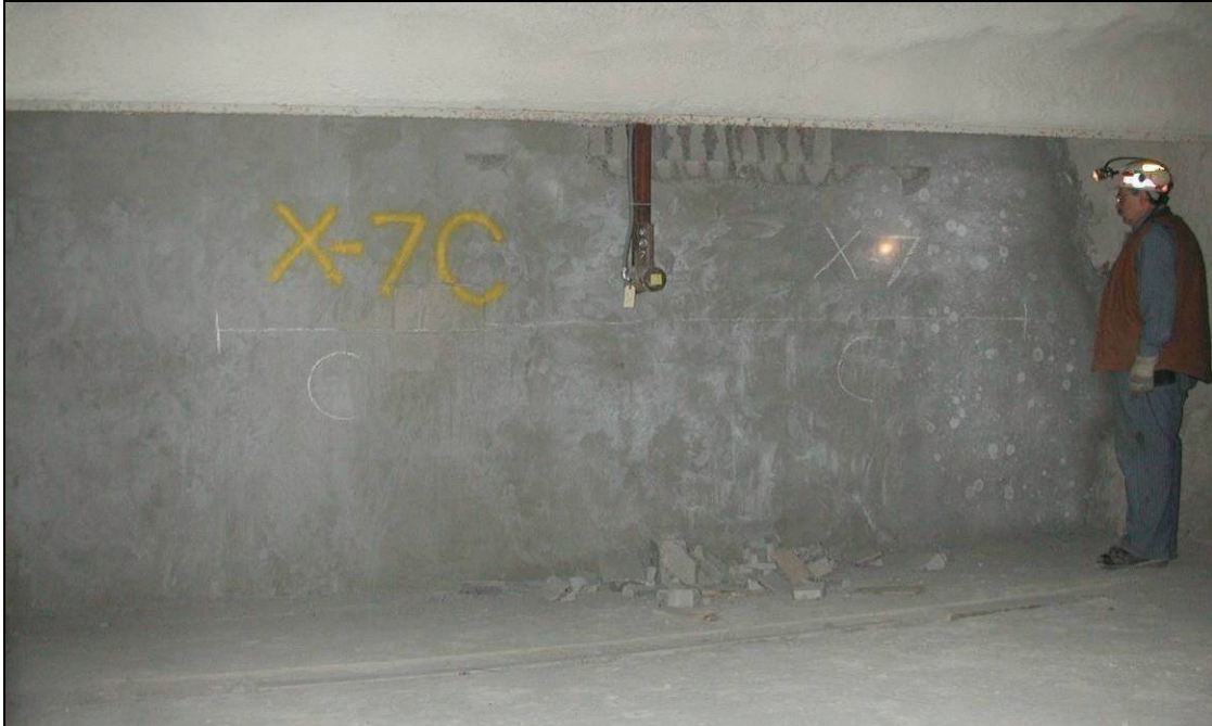
Figure 54.—Condition of X-7 dry-stacked hollow-core concrete block stopping after explosion test #433, viewed from C-drift side.
