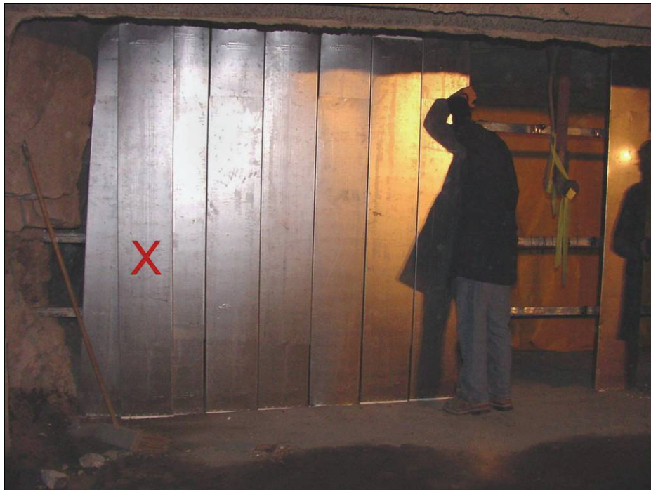
Figure 20.—Overlap panel (indicated by an “X”) used to close gap between rib panel and second panel, as viewed from the front or C-drift side.
