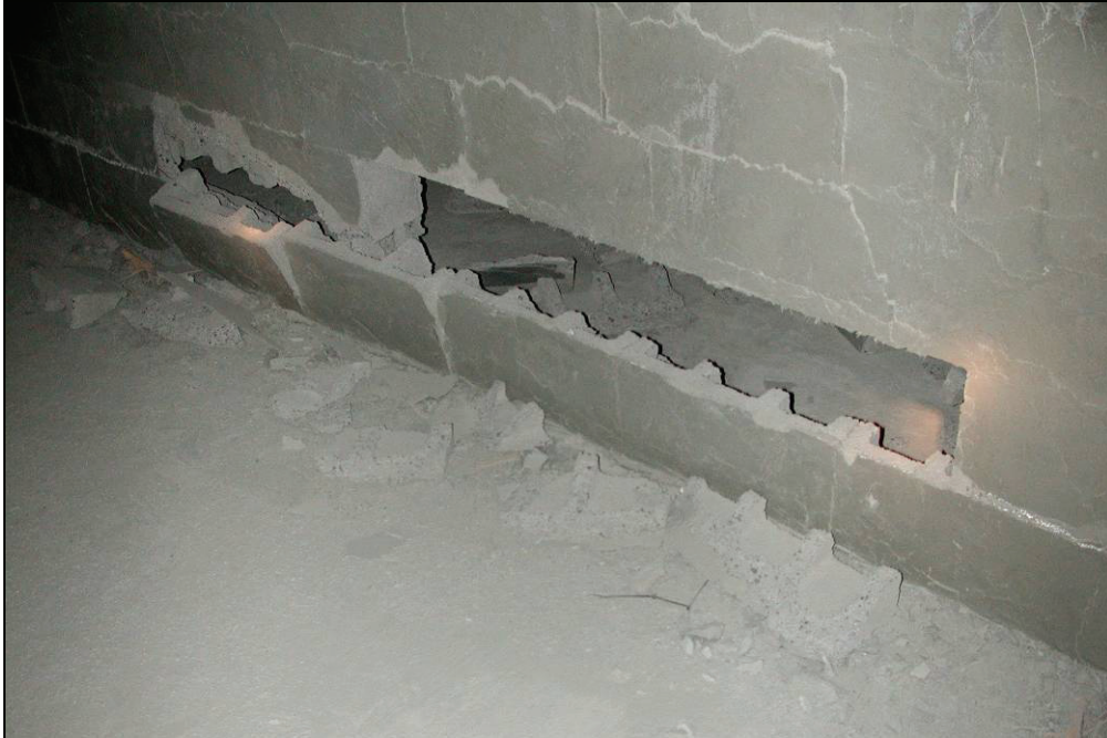
Figure 47.—Closeup of C-drift side X-6 dry-stacked hollow-core concrete block stopping after test #430, showing missing and damaged blocks.
