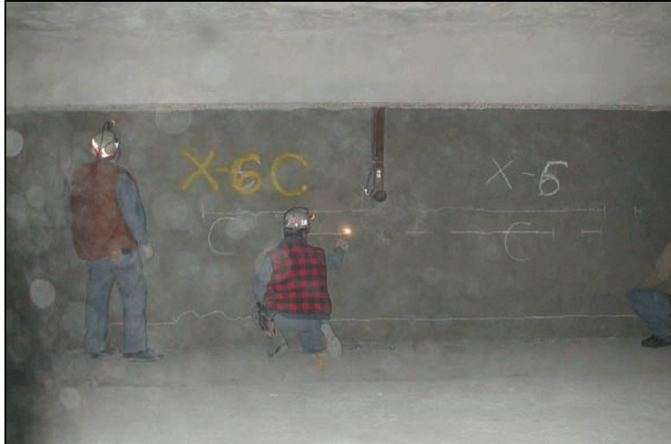
Figure 41.—Dry-stacked hollow-core concrete block stopping in X-6 remained intact after LLEM test #428. Chalk highlighted the cracks in the surface coating material.
