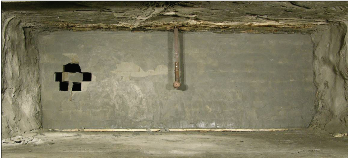
Figure 94.—Damage to the X-3 dry-stacked hollow-core concrete block stopping between B- and C-drifts after LLEM test #497.
