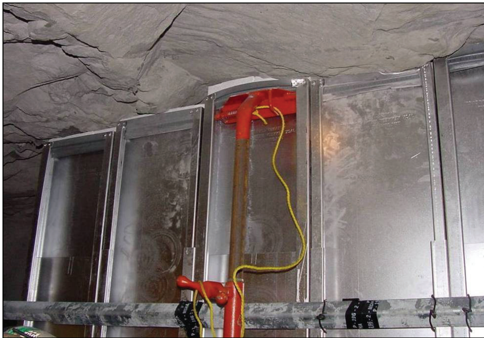
Figure 18.—Temporary jack used to exert roof-to-floor pressure on the metal panel during installation.
