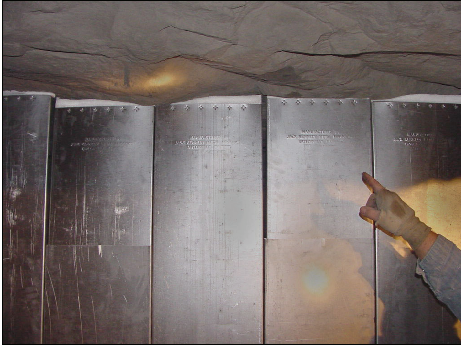
Figure 17.—Polystyrene foam head seal used to provide enhanced closure between metal panel and roof, as viewed from the C-drift side.
