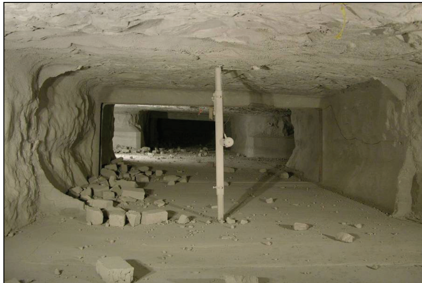
Figure 84.—Debris from 6-in (15-cm) thick, wet-laid solid block stopping in X-7 after LLEM test #519, viewed from A-drift.
