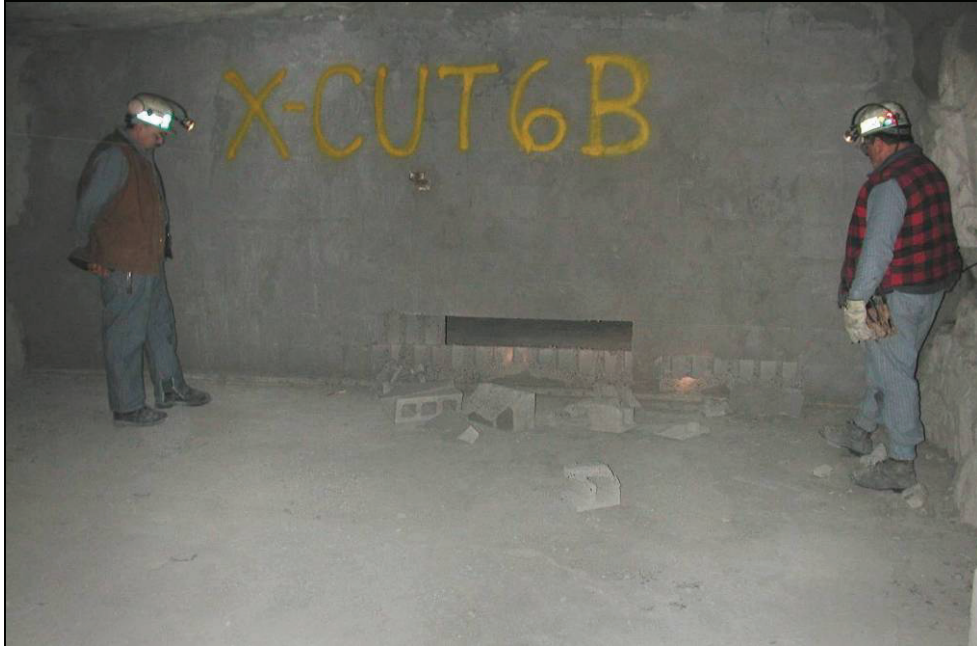
Figure 45.—Crosscut 6 dry-stacked hollow-core concrete block stopping viewed from B-drift side after LLEM test #430, showing blocks dislodged by explosion.
