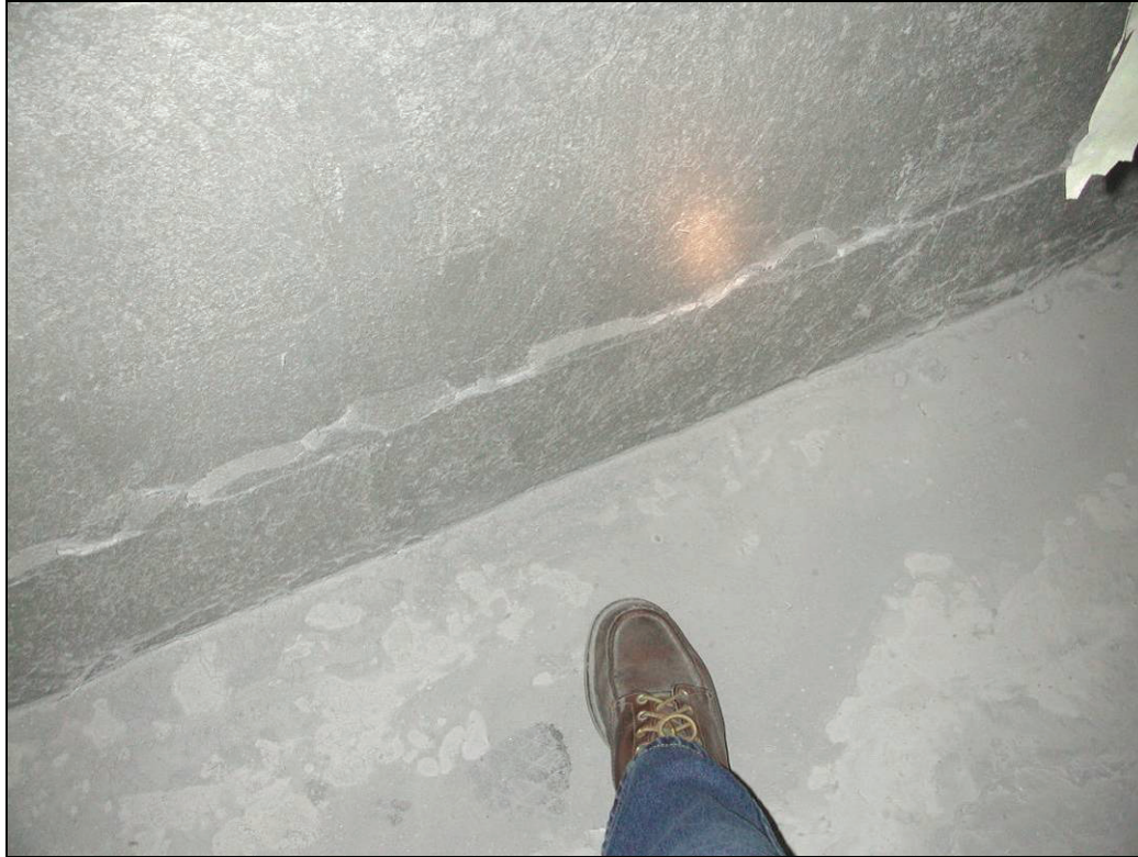
Figure 70.—Displacement of the second block course at the X-4 dry-stacked solid-concrete-block stopping after LLEM test #459, viewed from C-drift.
