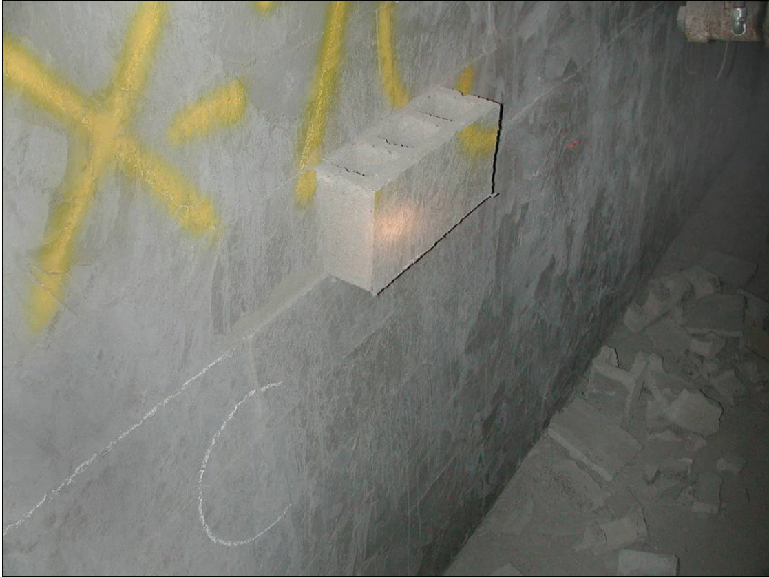
Figure 56.—Expanded view of hollow-core concrete block that is almost dislodged from X-7 dry-stacked stopping after explosion test #433.
