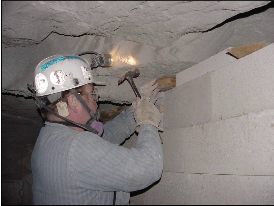
Figure 6.—Installation of wood header boards and wood wedges between the stopping and roof for dry-stacked hollow-core concrete block stopping.
