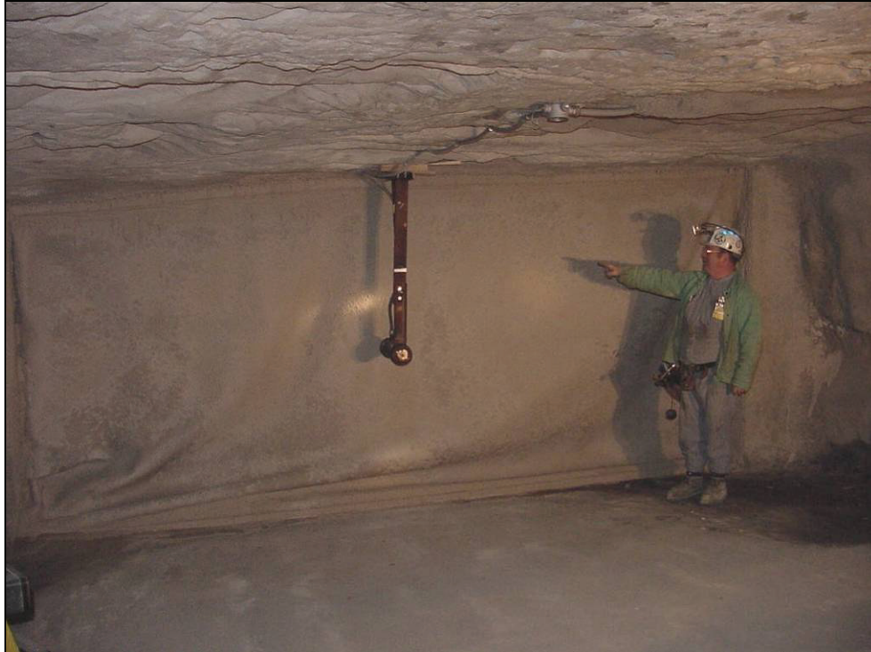
Figure 31.—Completed woven cloth stopping design in X-6, viewed from the explosion or C-drift side.
