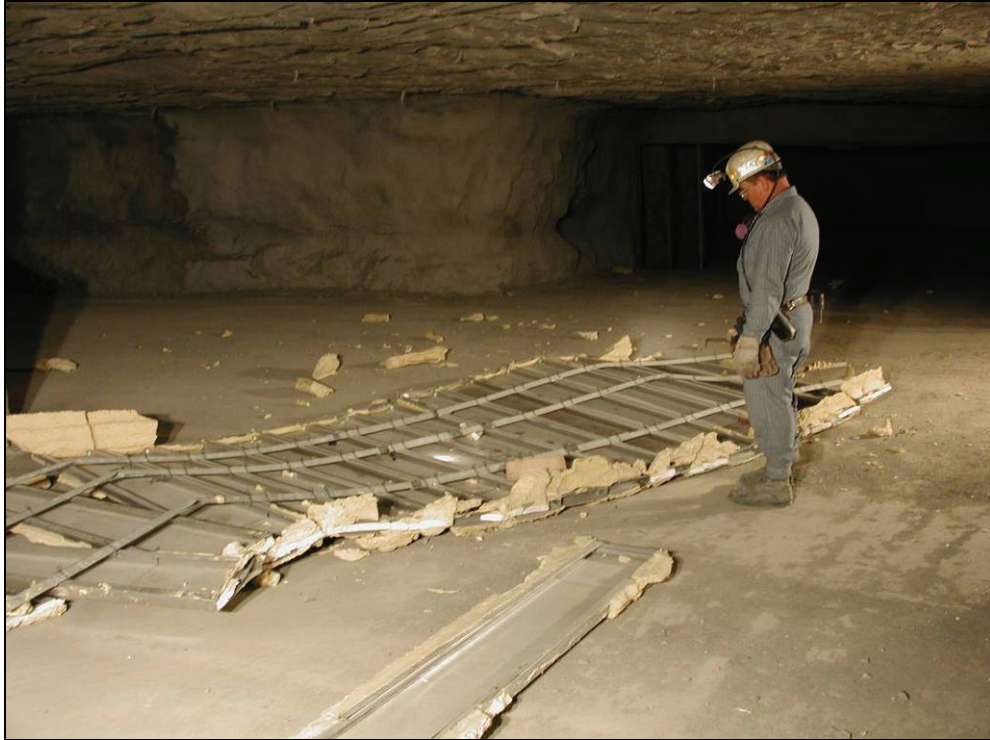
Figure 63.—Debris from steel panel stopping in X-6 after LLEM test #458, viewed from C-drift.
