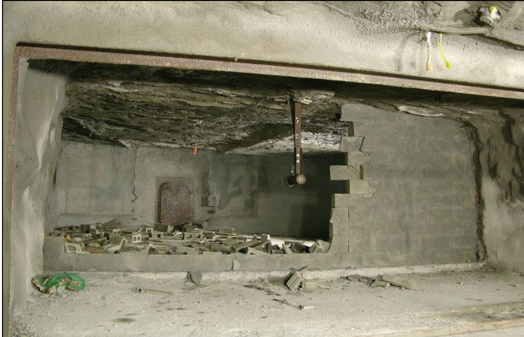
Figure 91.—Damage to the X-4 dry-stacked hollow-core concrete block stopping between B- and C-drifts after LLEM test #497.
