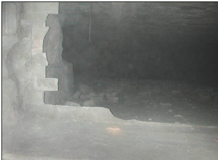
Figure 72.—Debris from the dry-stacked solid-concrete-block stopping and remaining blocks on the outby rib line in X-4 after LLEM test #462, viewed from C-drift.
