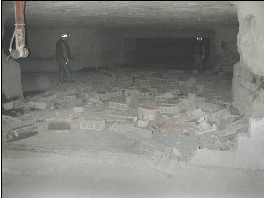
Figure 37.—Debris from X-5 dry-stacked hollow-core concrete block stopping after LLEM test #428, viewed from C-drift.
