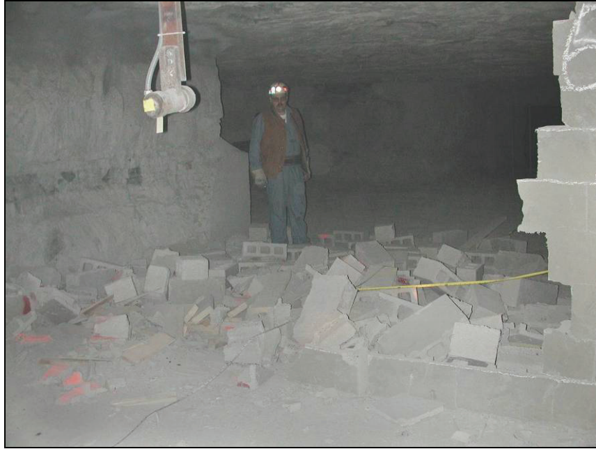
Figure 50.—Debris from X-6 dry-stacked hollow-core concrete block stopping after LLEM test #433, viewed from C-drift.
