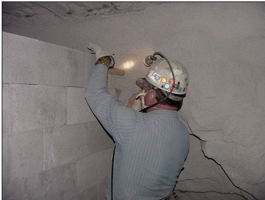
Figure 5.—Installation of wood wedges between the stopping and rib for dry-stacked hollow-core concrete block stopping.
