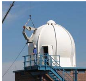
Out with the old and in with the new, here is the new RRS antenna being installed within the domed upper air building at the NWS Spokane office.
