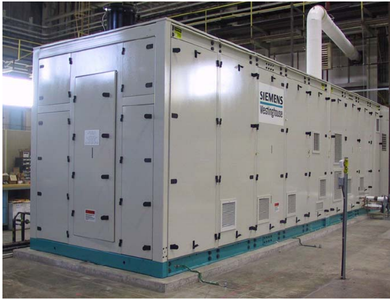
Figure 7-28 Siemens Westinghouse 250 kW Tubular SOFC Installation (31)
