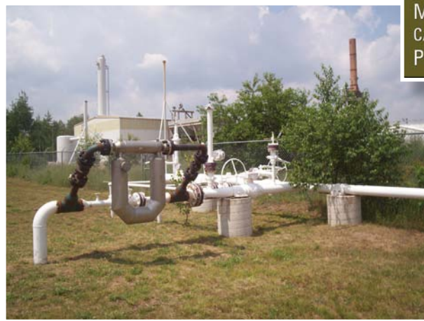
CO 2 pipeline from a gas processing plant in Michigan.
