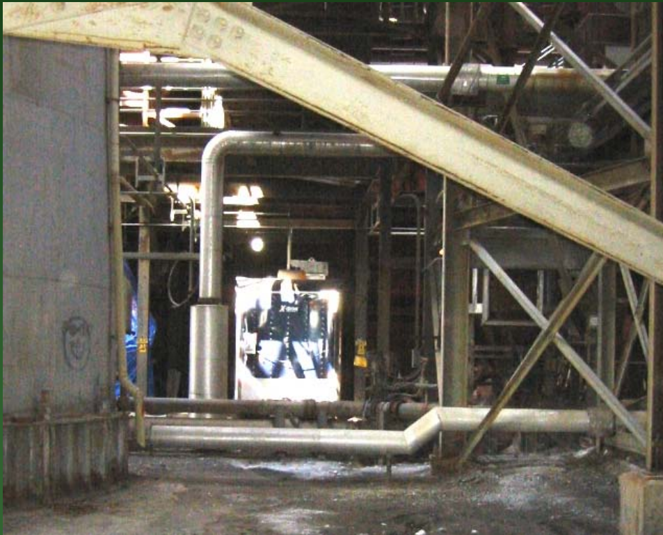
Mobile injection trailer (patent pending) in place.
