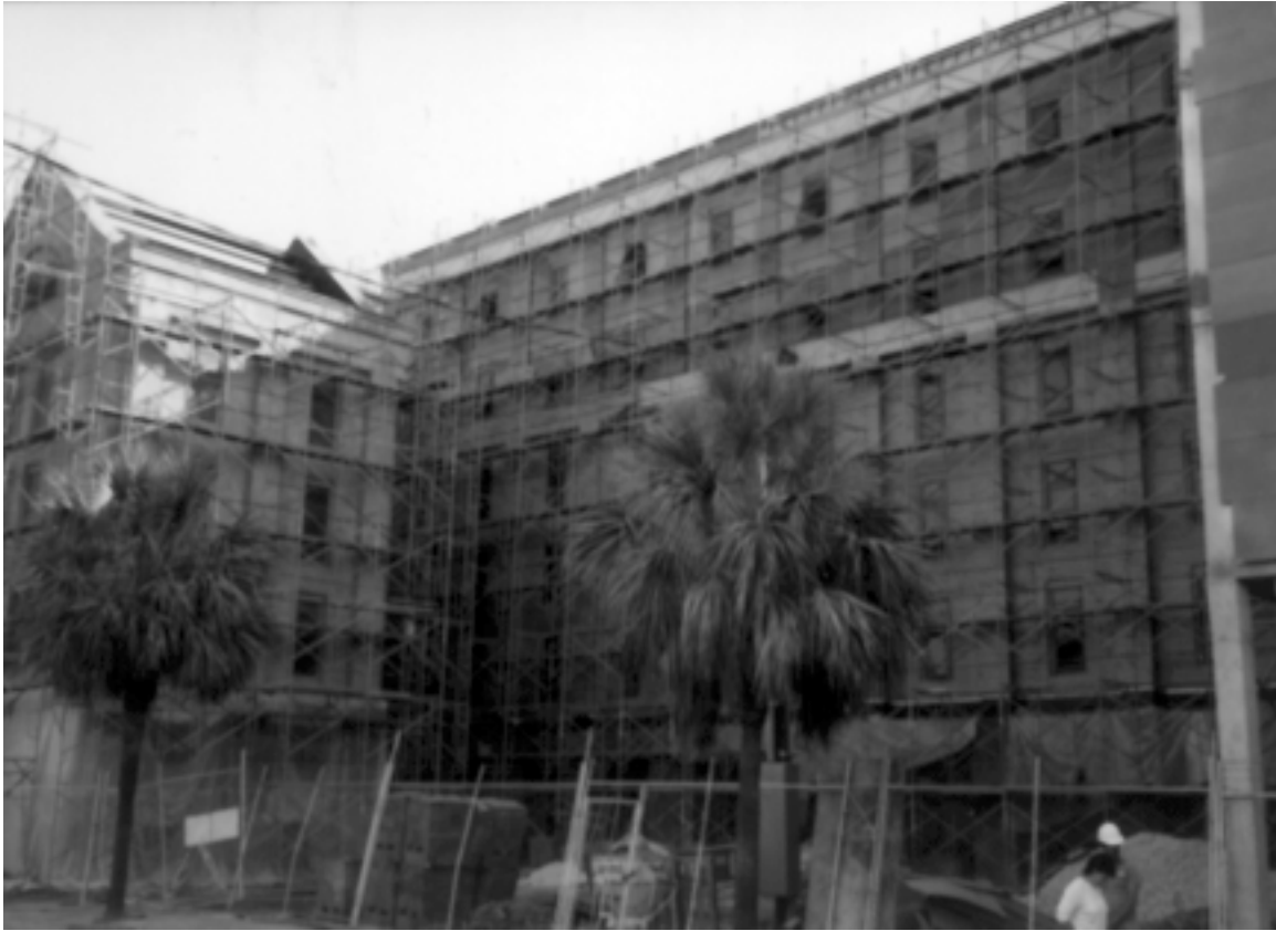
Figure. The victim fell from the fifth-floor level of the scaffolding shown here, when he either stood on or fell against the guardrail causing it to give way. The victim was not wearing any fall protection equipment.
