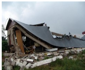
Damage from an EF1 tornado. CASA graduate student Patrick Marsh (University of Oklahoma) conducted a damage survey to verify the EF1 tornado identified in CASA data. Credit: CASA.
