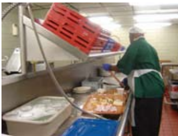
Photo 1: Mechanical Dishwashing Table. The trays cover the table's drain. On the far left side of the photo is the pulper.
