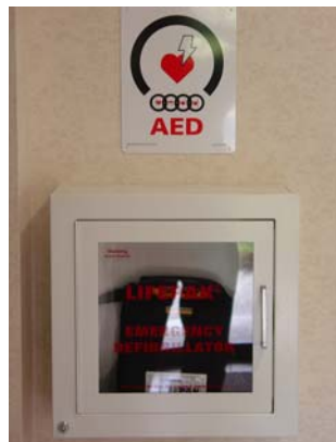
AED located in the lobby of the main office
