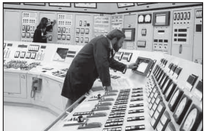
FFTF control room.
