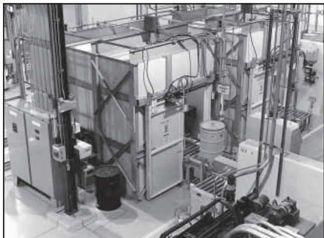
An analytical cell inside the Waste Receiving and Processing Facility.
