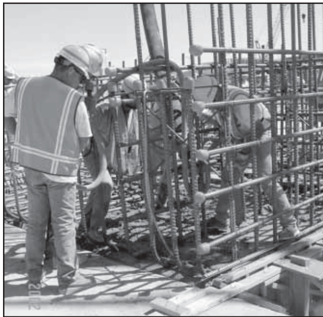
Workers place the first structural steel in the high-level waste treatment facility.
