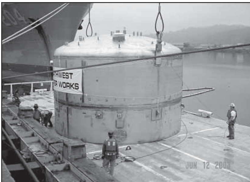
Pressure vessel for the pre-treatment facility.
