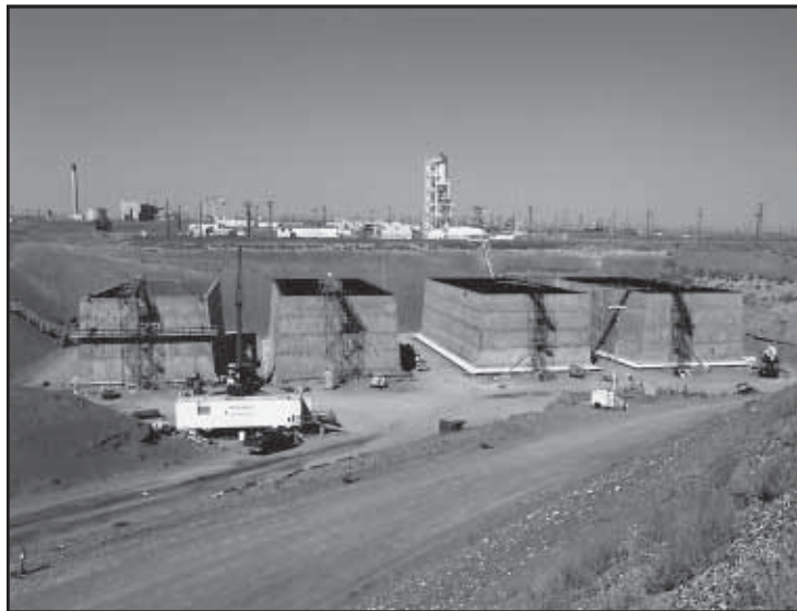
Grout vaults under construction — the grout program was abandoned as part of a TPA renegotiation.
