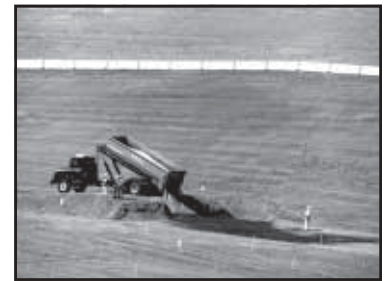
The first load of waste is dumped at Hanford’s Environmental Restoration and Disposal Facility.
