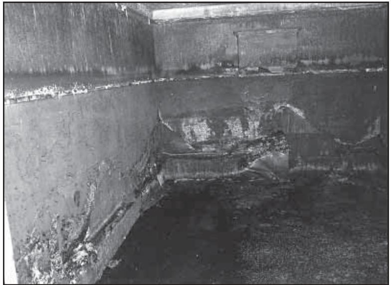
The view inside Tank 241-Z-361.
