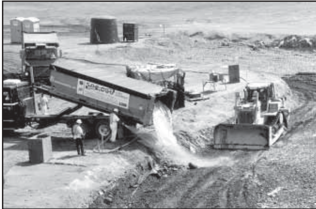
The one millionth ton of contaminated material is dumped at Hanford’s ERDF.
