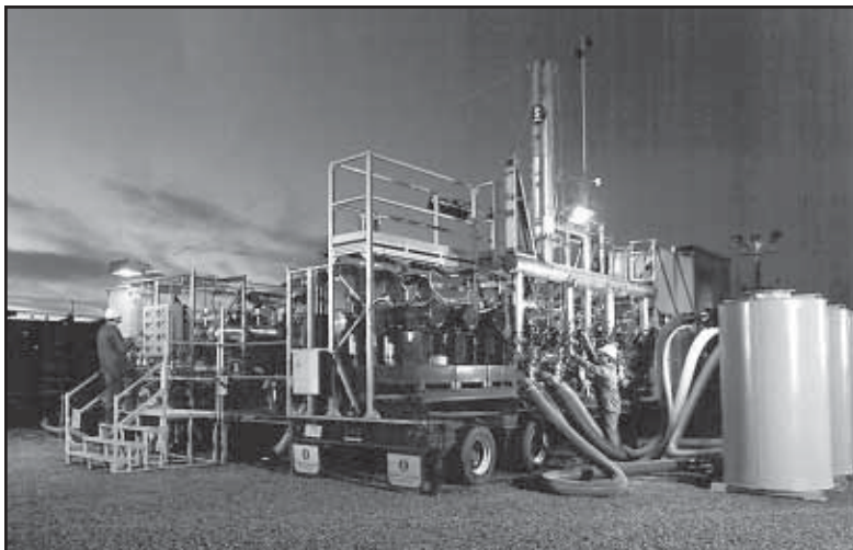
Carbon tetrachloride vapor extraction system.
