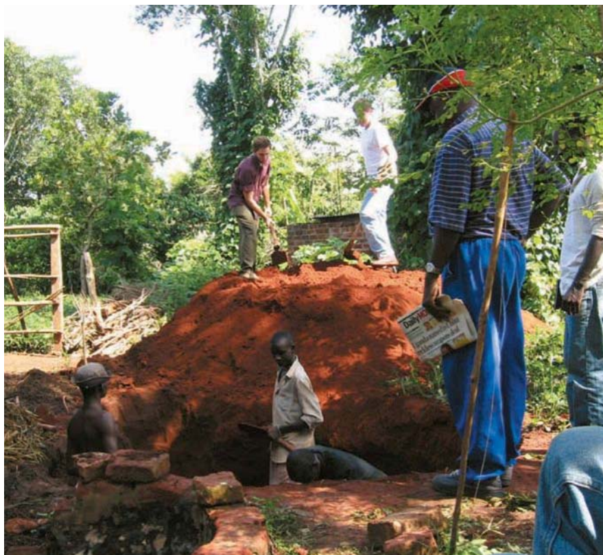
...and then work with Ugandans to dig a pit for the digester.
