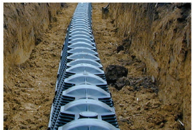
Figure 3. Drainfield with chamber prior to backfilling with soil for a gravelless system.
