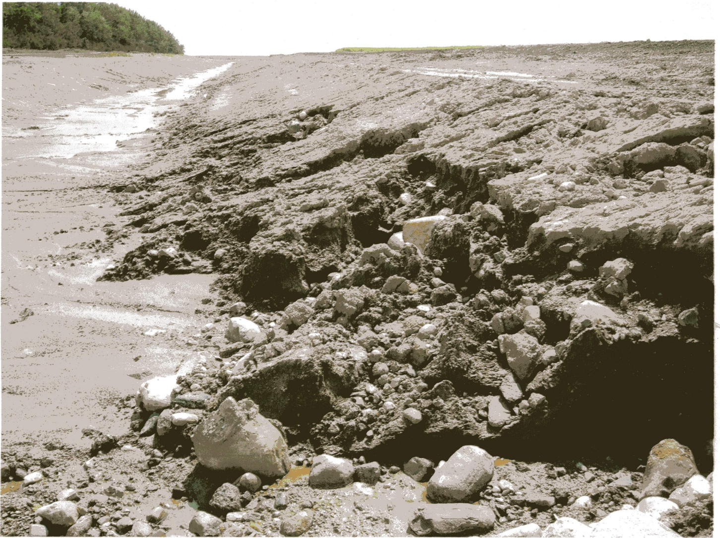
Figure 1. Fissures and/or blow-outs & cobbles (larger than 3") on James Elstad properties, NW1/4, Section 9, T151N R68W, Benson County, ND along the inside portion of the Devils Lake Emergency Outlet Project.
