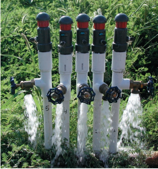
Figure 6. Flushing an SDI system.
