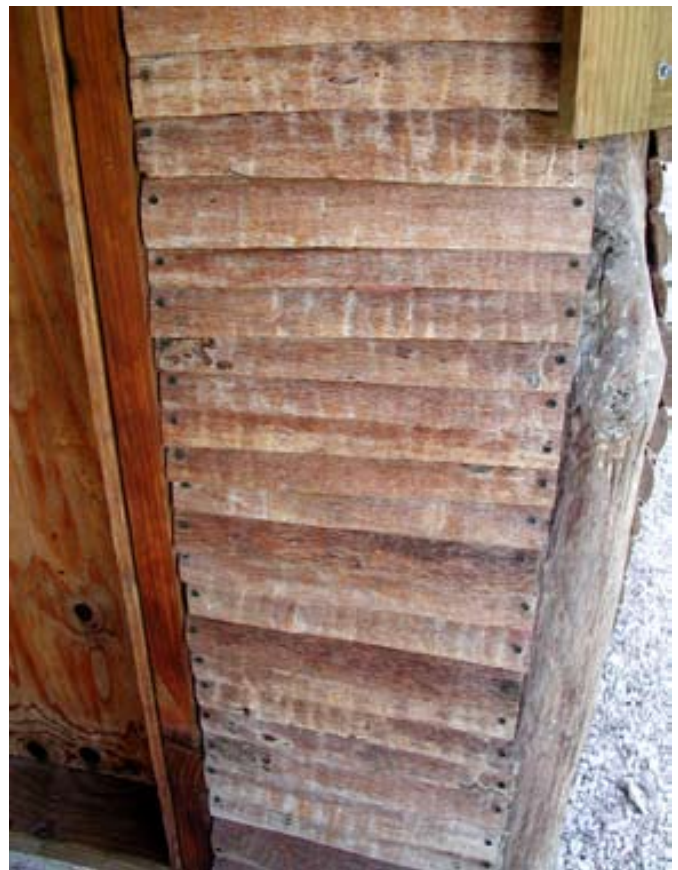
Top: Thatch wall. Bottom: House side panel made of pandanus slats. PHOTOS: L. THOMSON
